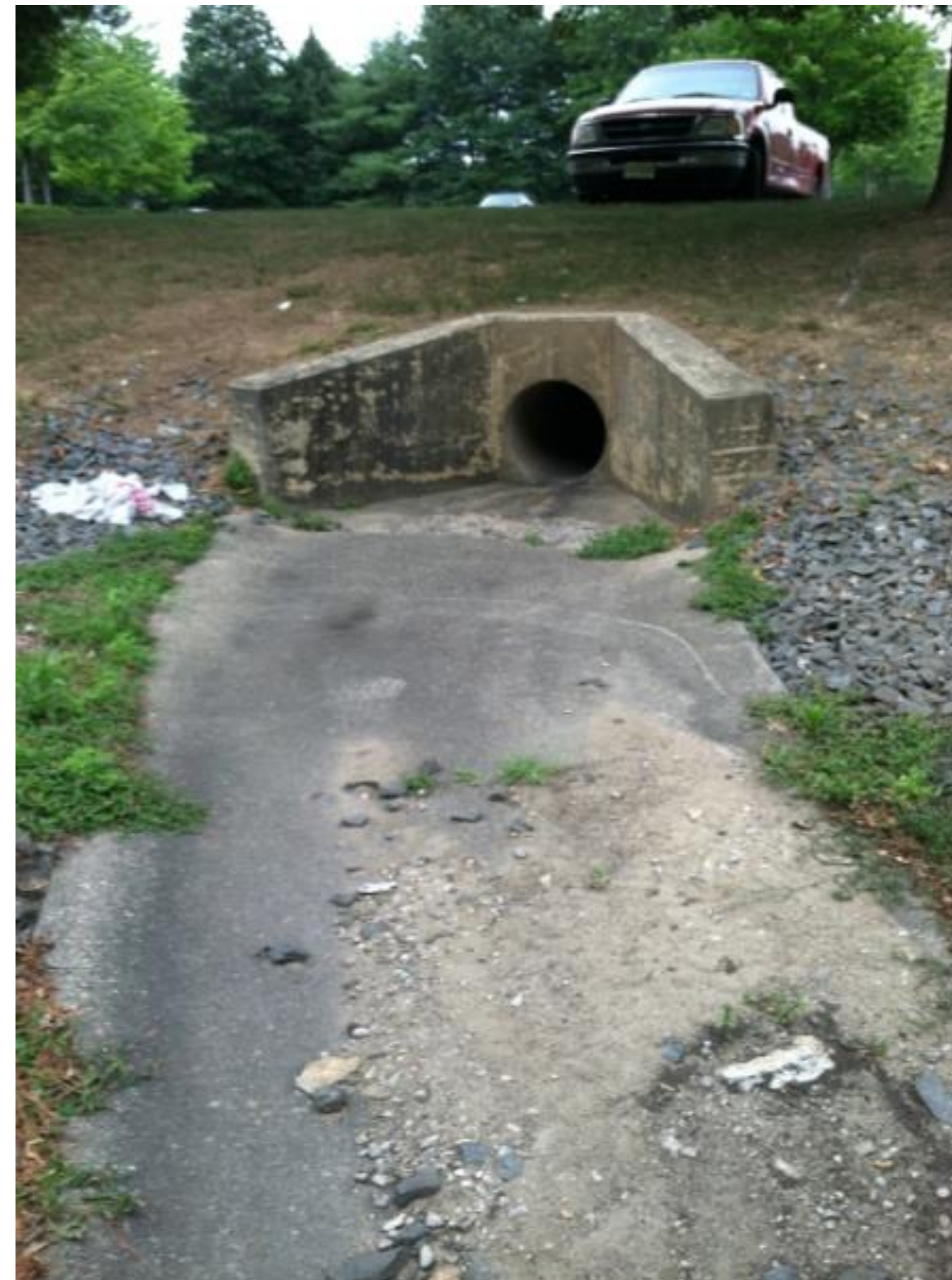
Inlet, sediment in low flow channel
