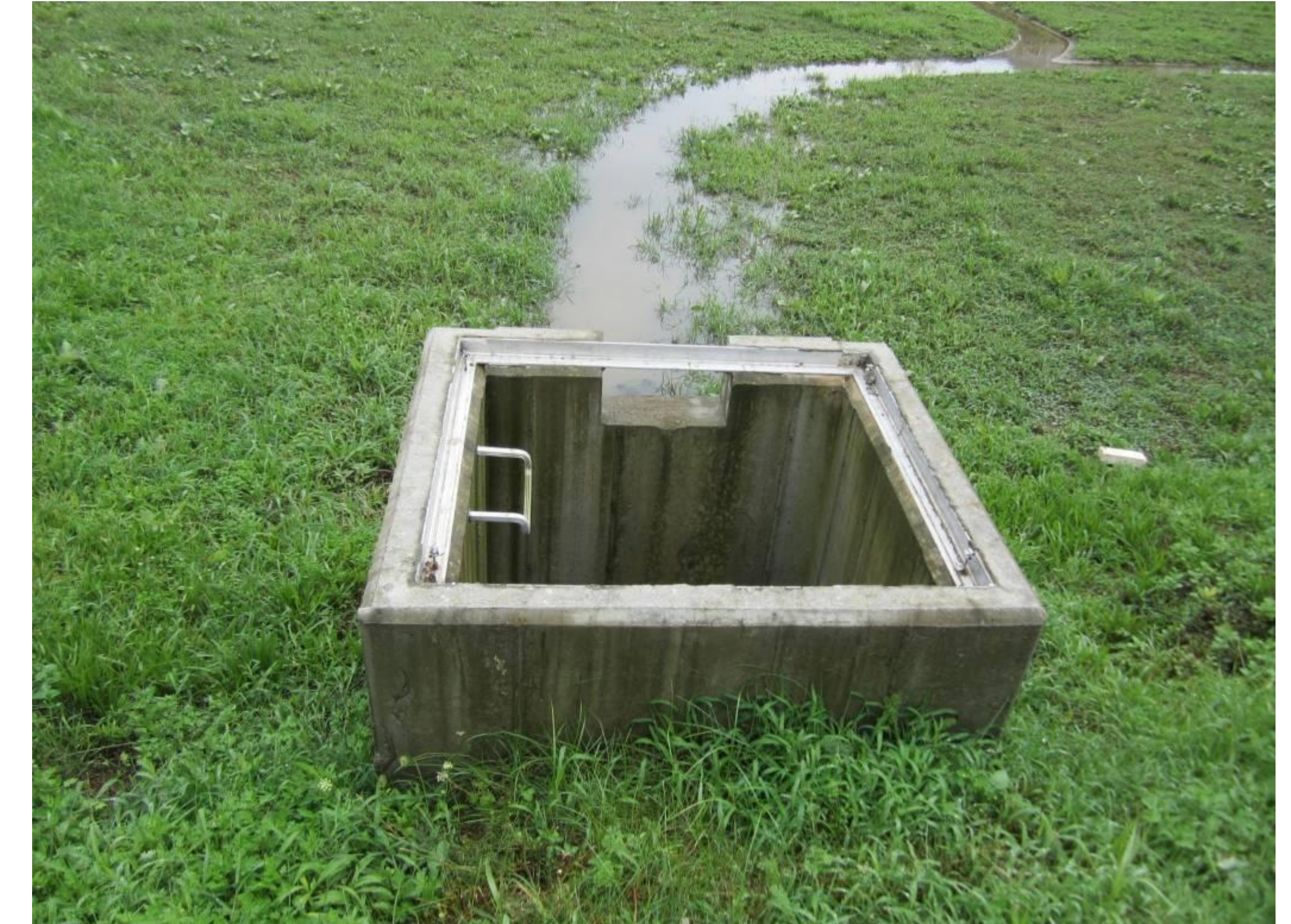
Outlet structure missing grate
