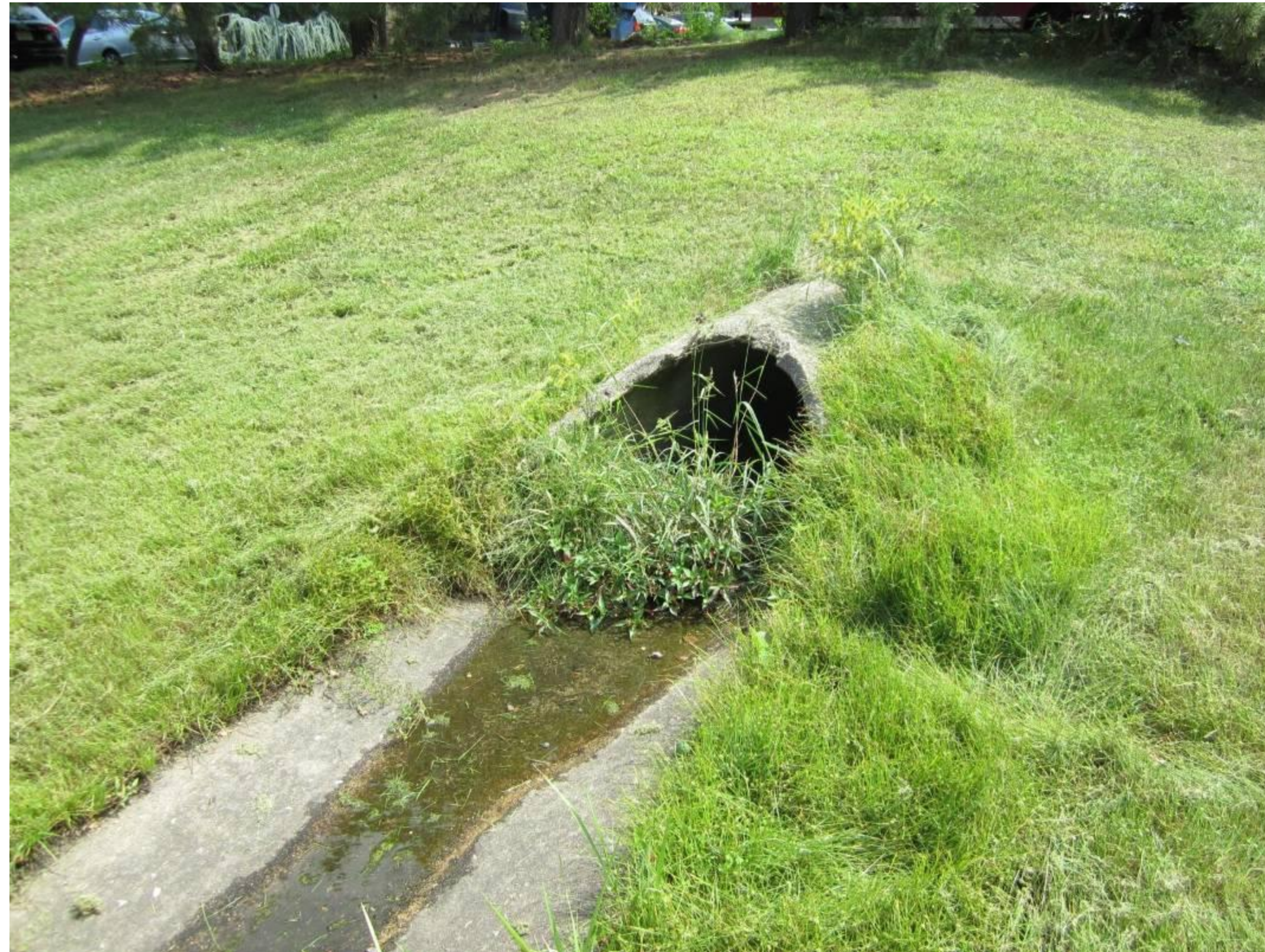
Excess sediment accumulation at inlet
