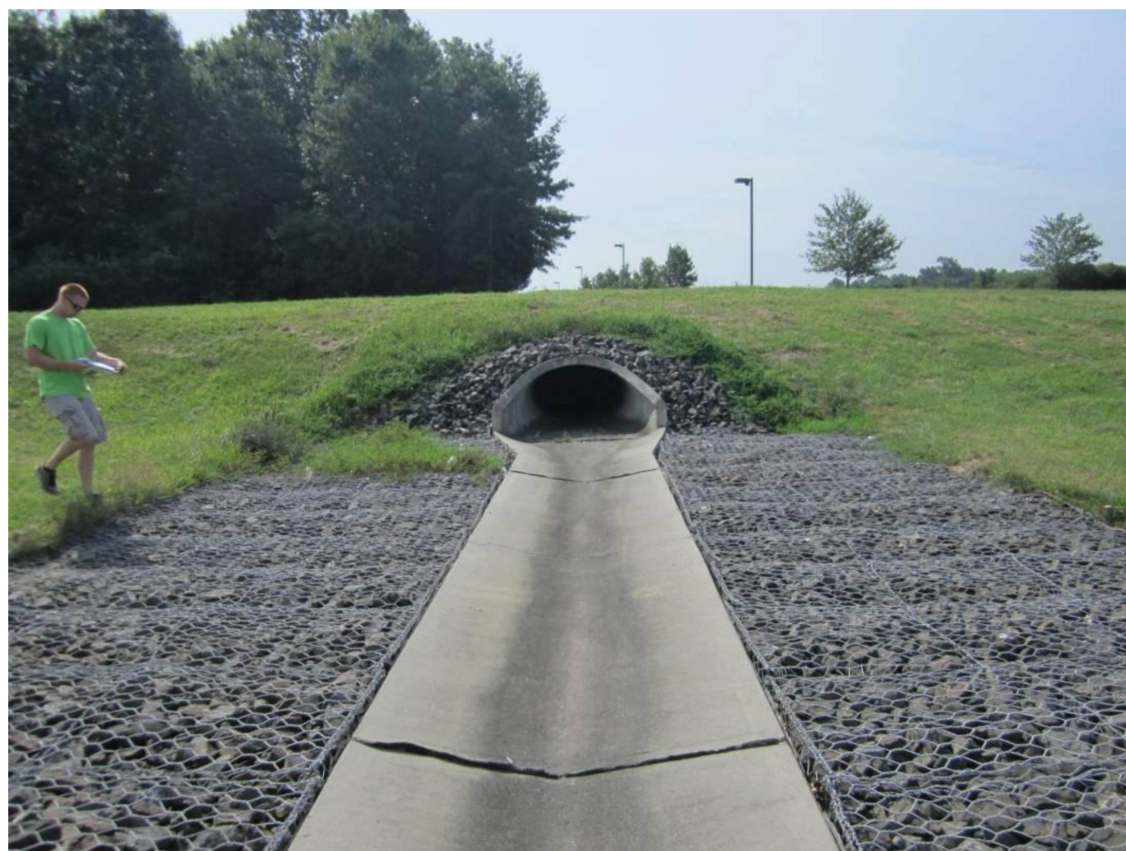
Inlet and rip rap protection
