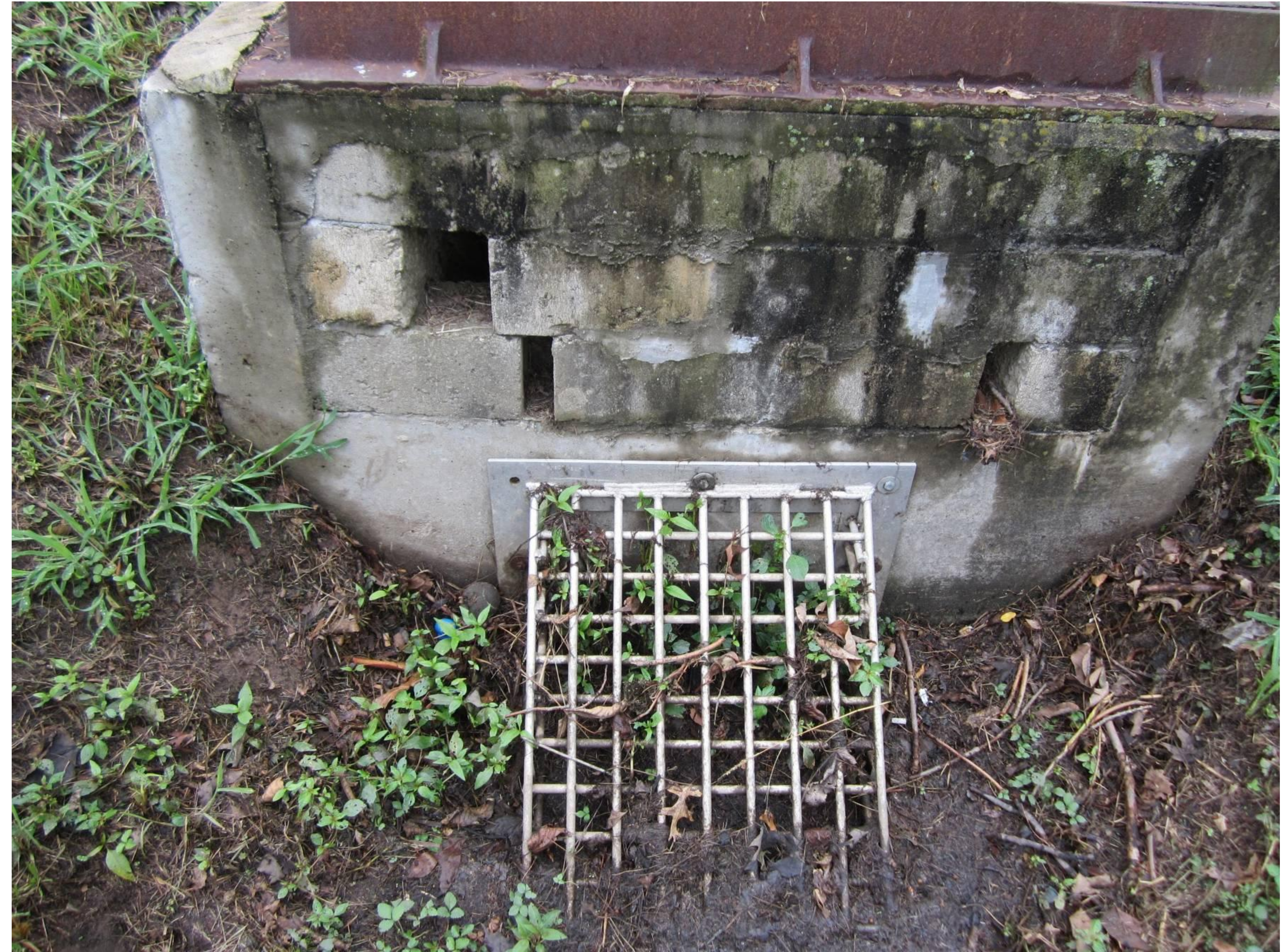
Clogged trash rack at outlet
