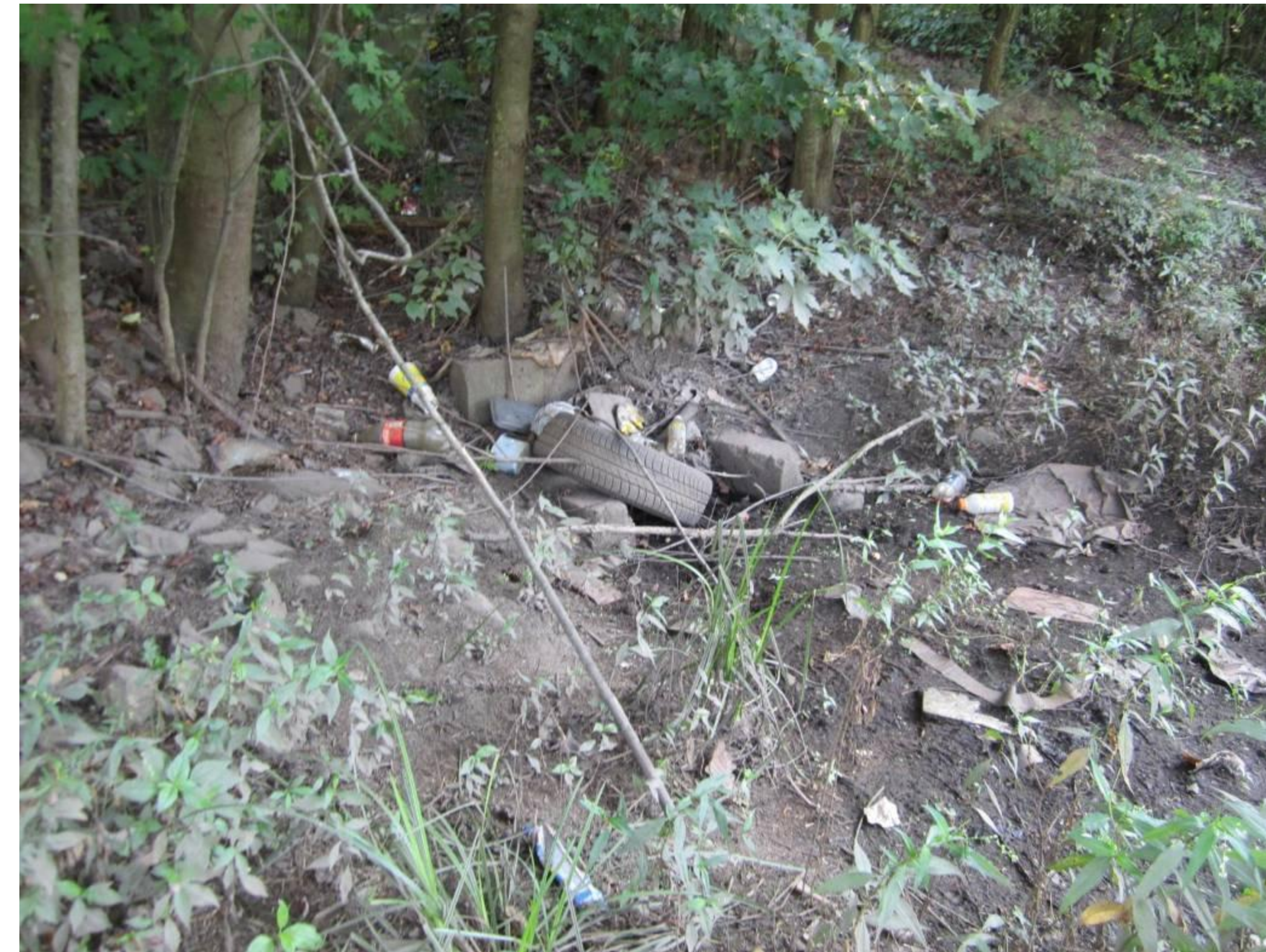
Outlet structure obstructed with litter
