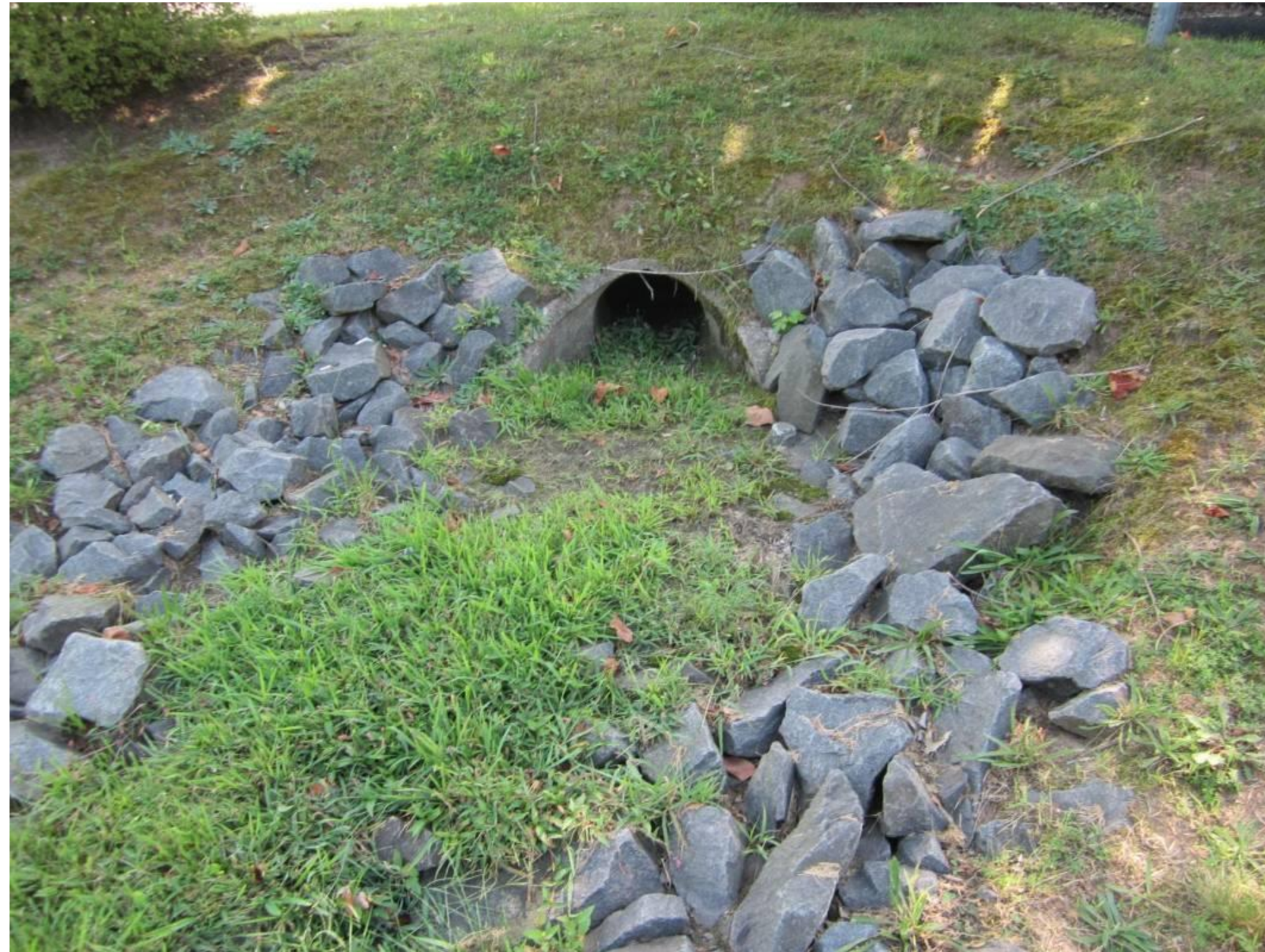
Inlet with sediment accumulation
