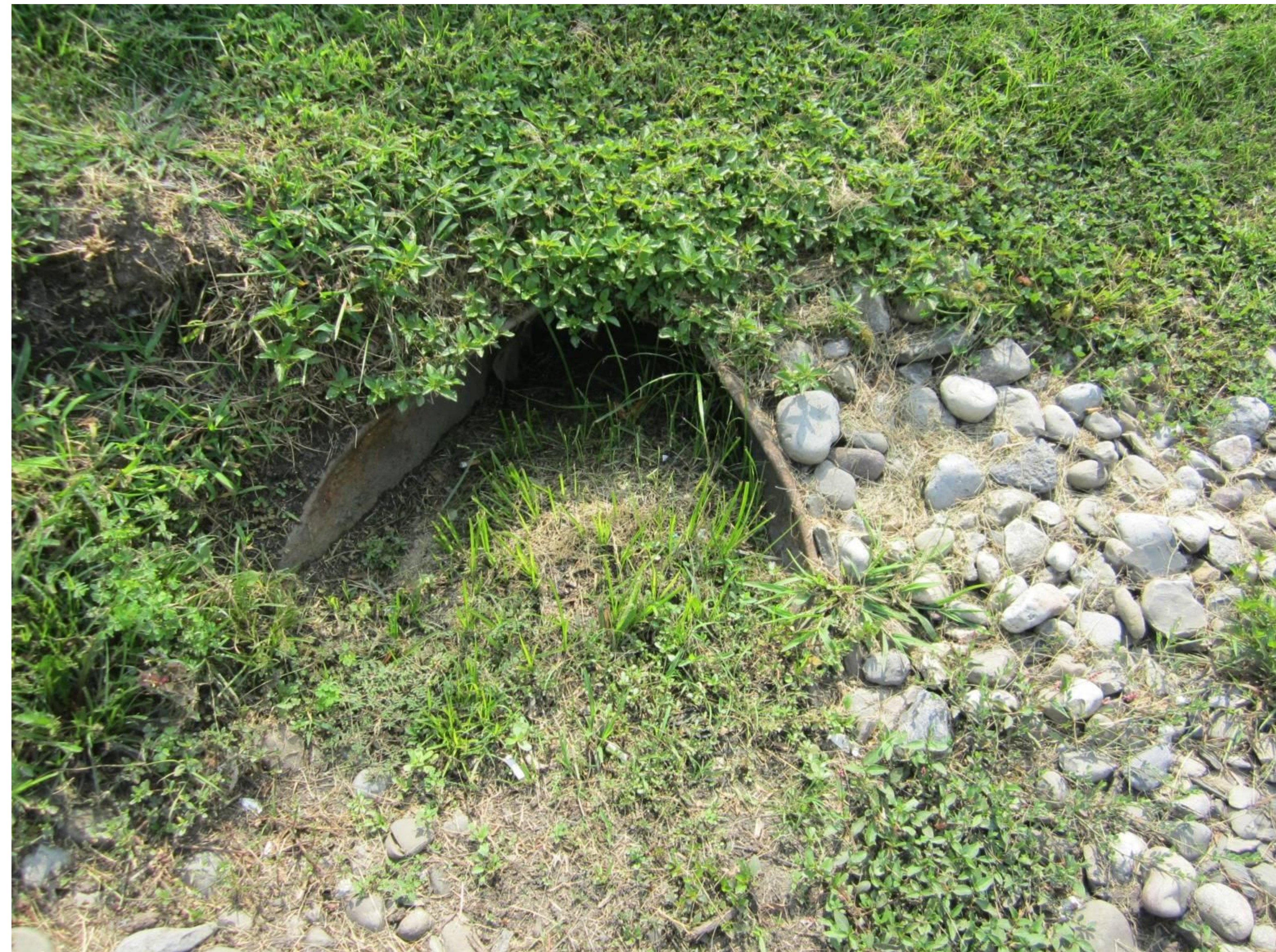
Sediment accumulation in inlet
