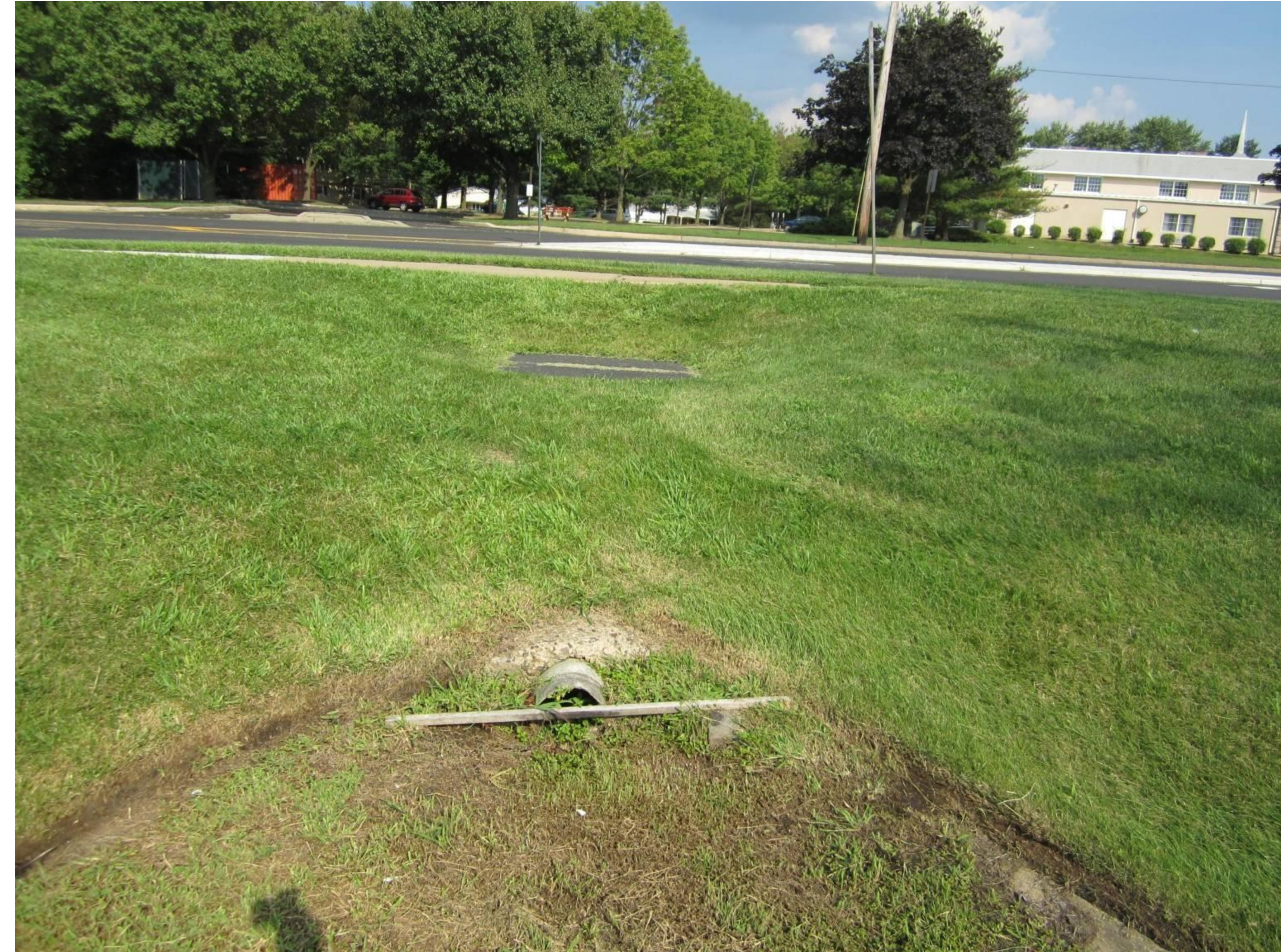
Outlet pipe and overflow
