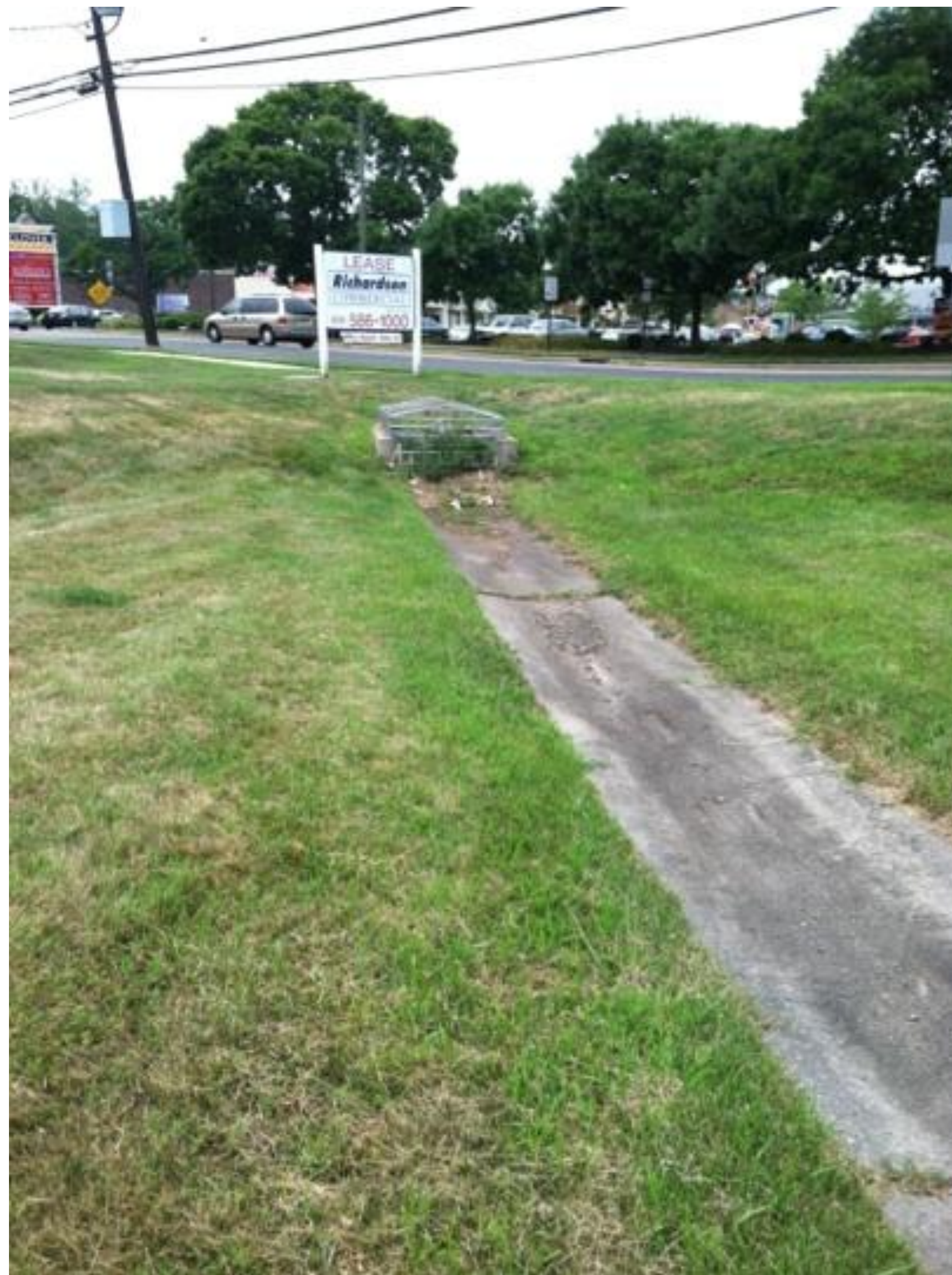
Low flow channel and clogged outlet
