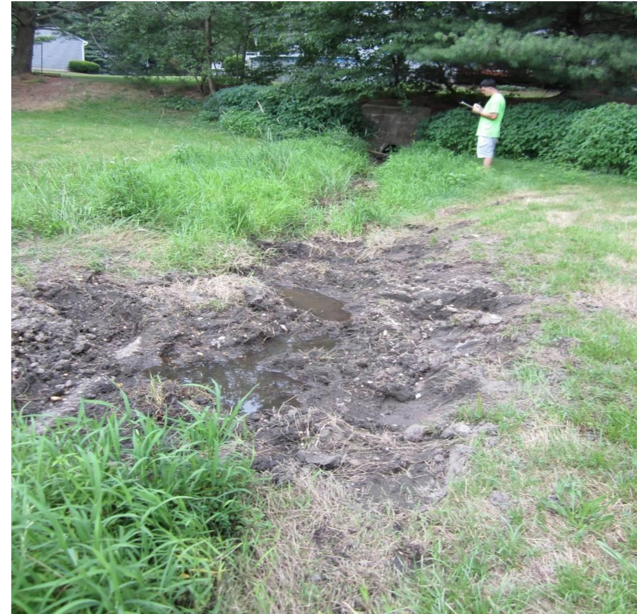
Clogged low flow and outlet.
