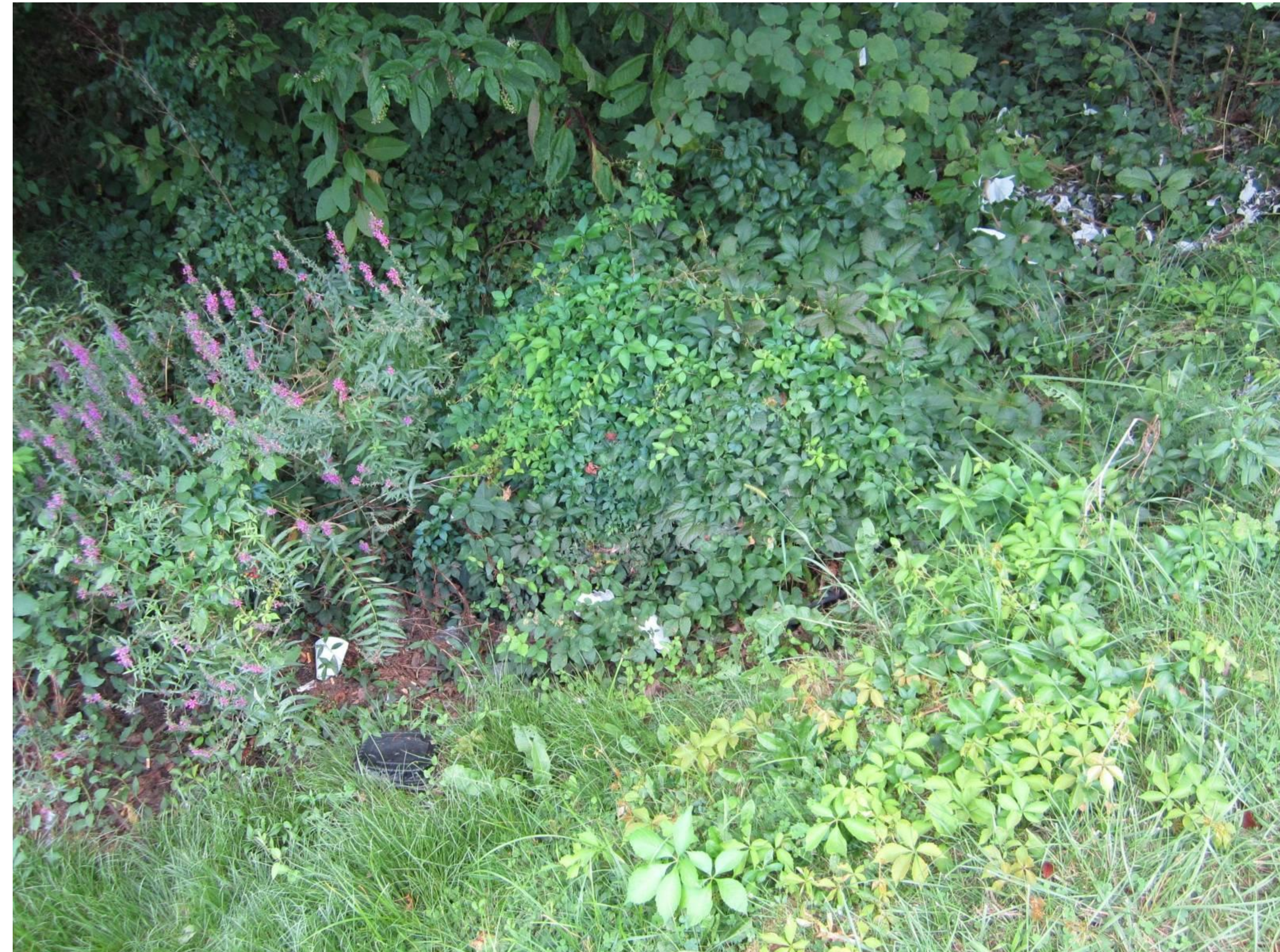
Excessive vegetative growth at outlet
