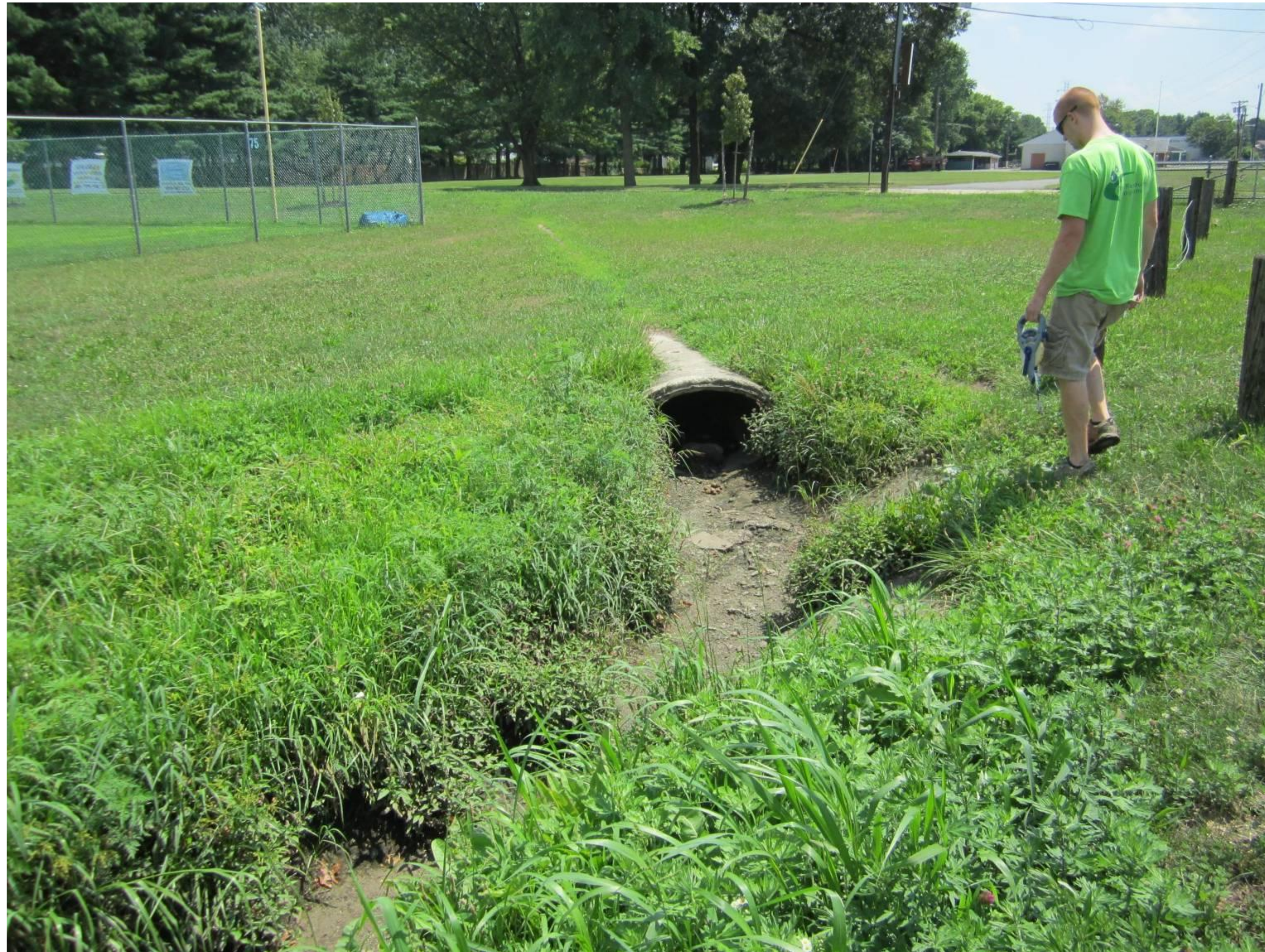
Inlet with sediment accumulation
