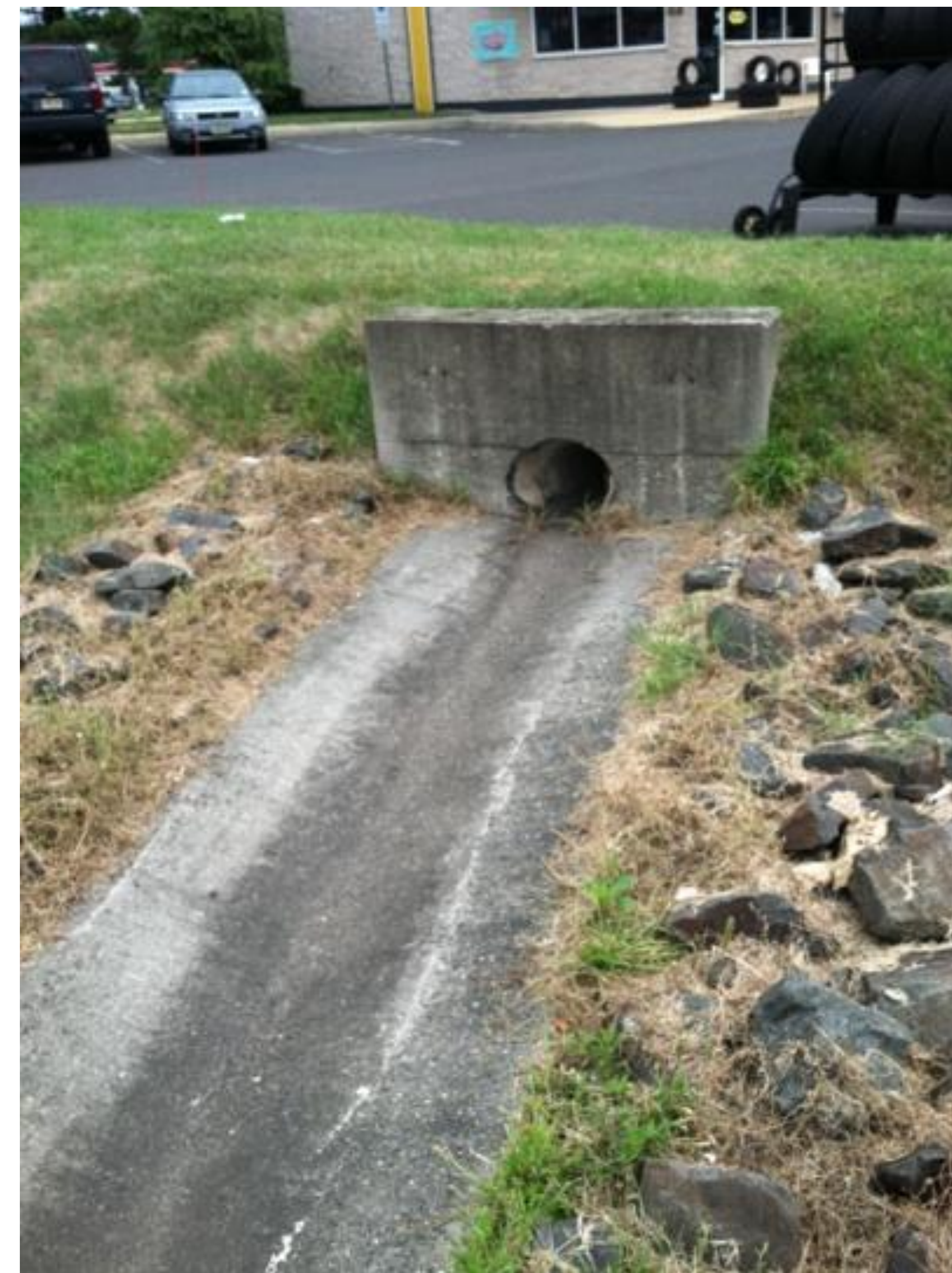
Inlet and rip rap protection
