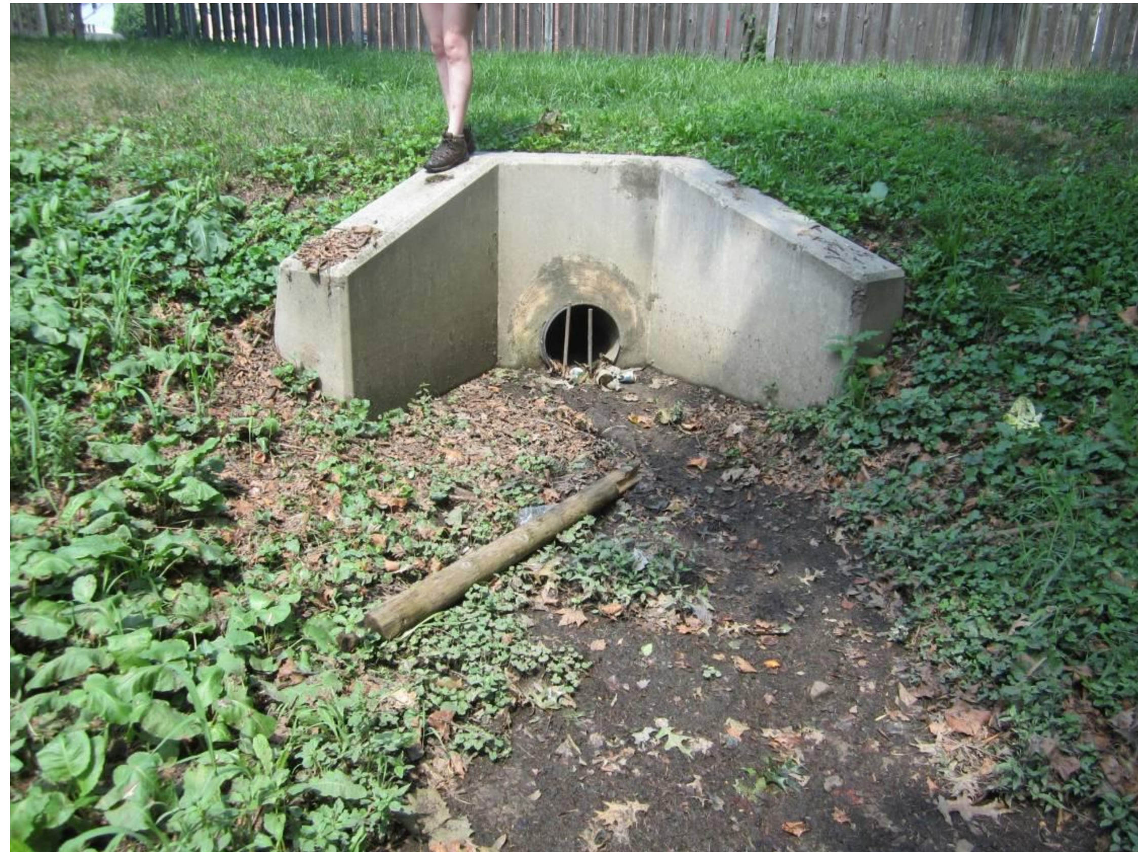
Inlet clogged with sediment
