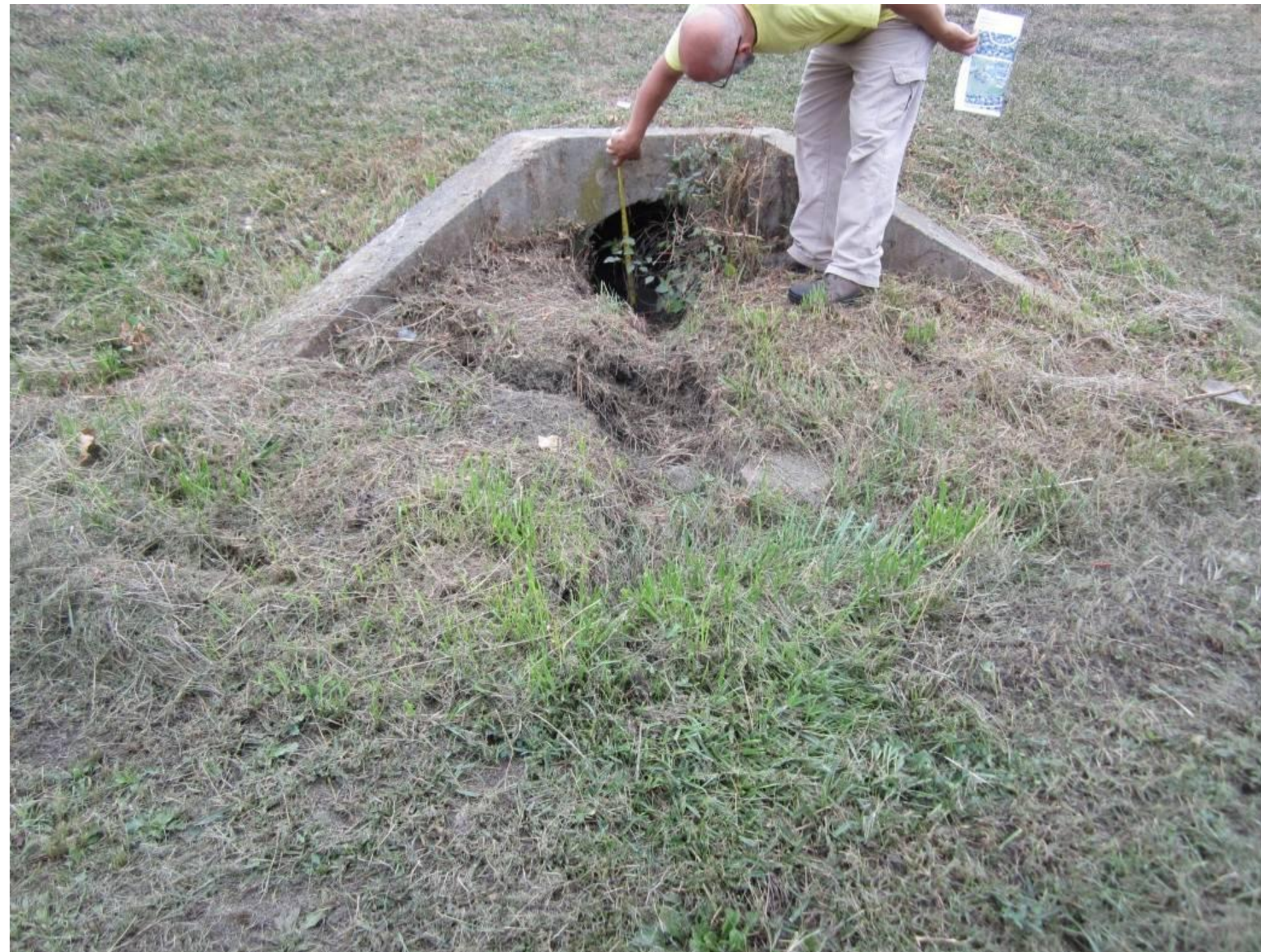
Sediment accumulation in the inlet
