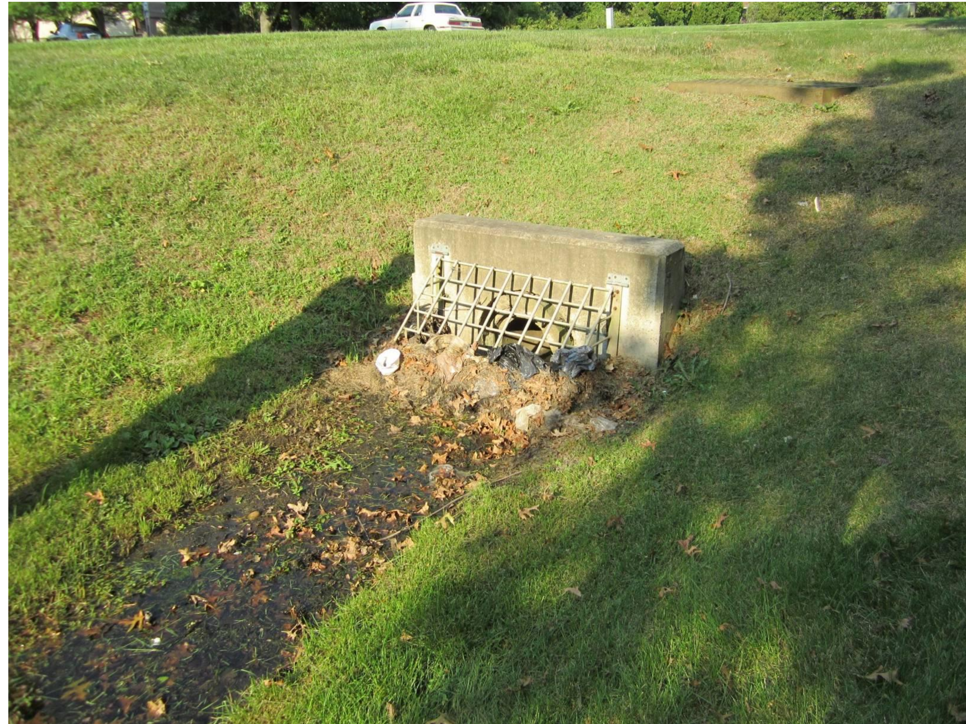
Outlet with clogged trash rack
