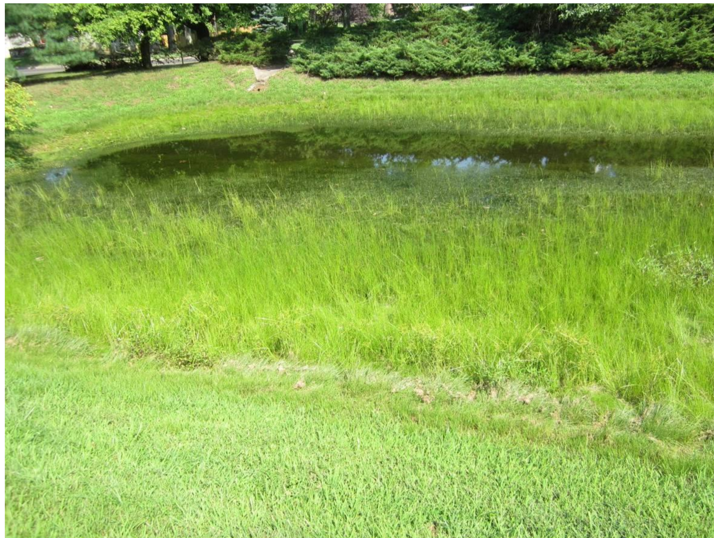
Ponding in basin bottom
