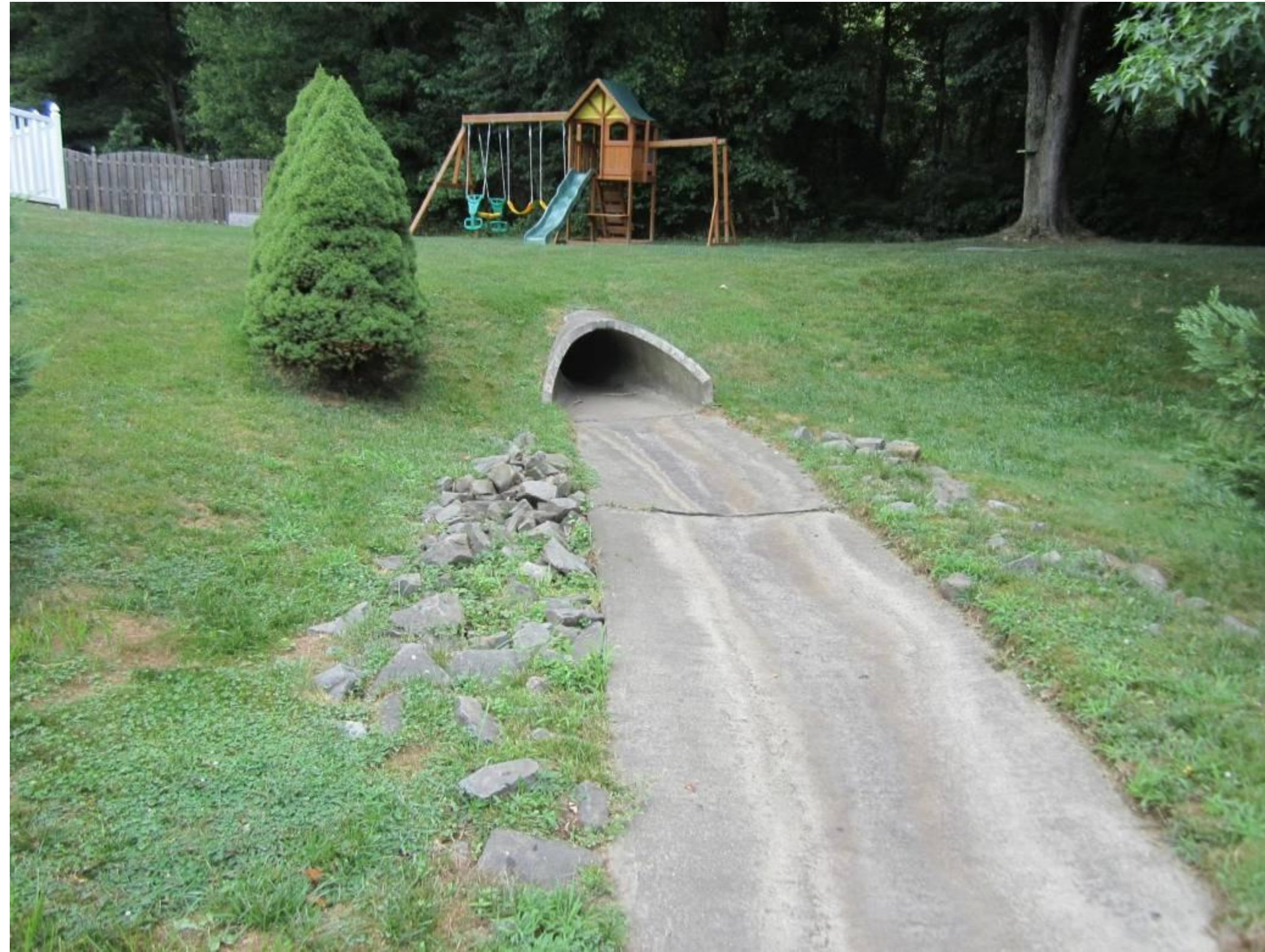
Inlet and low flow channel
