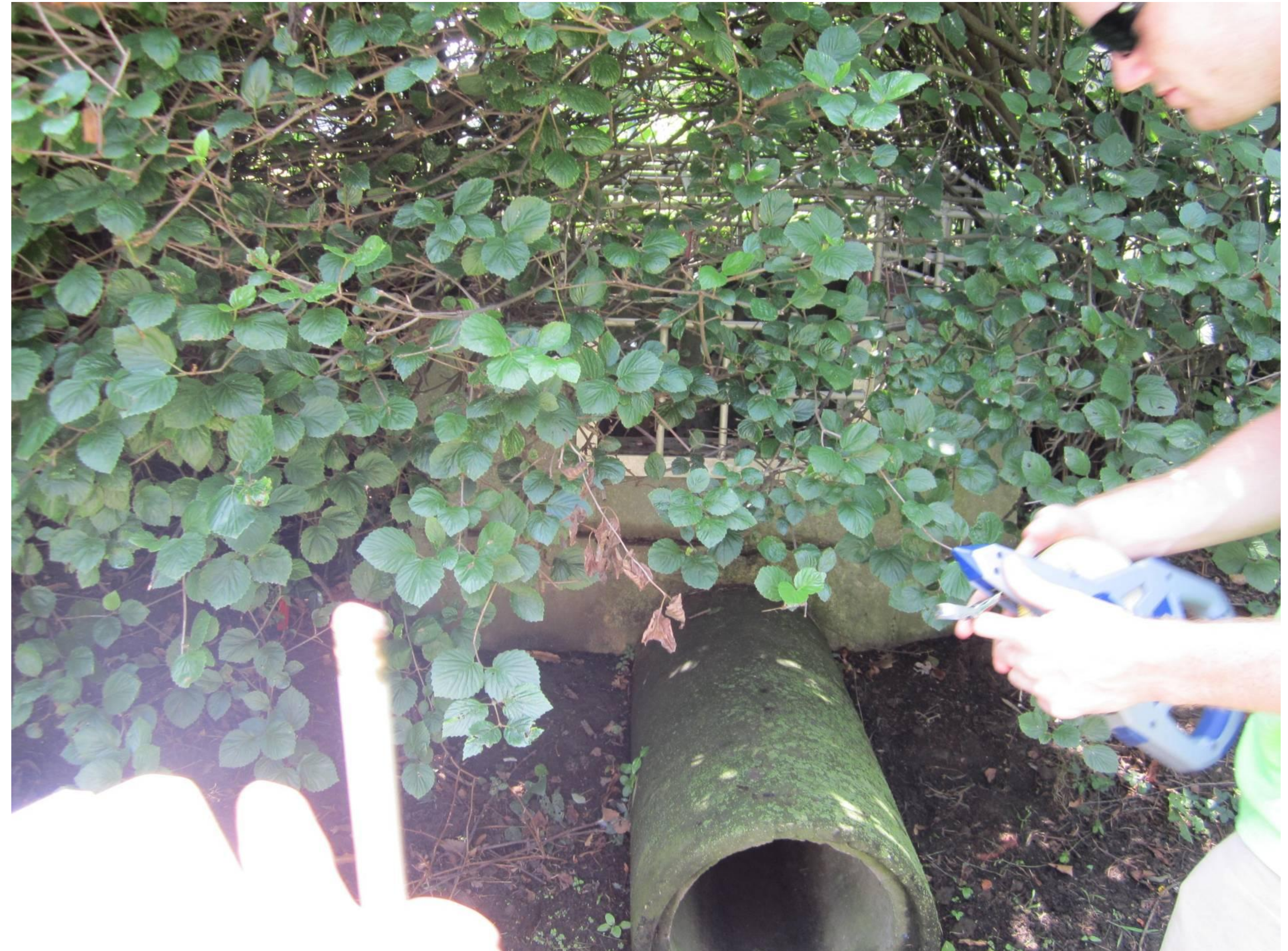
Woody vegetation growth around outlet
