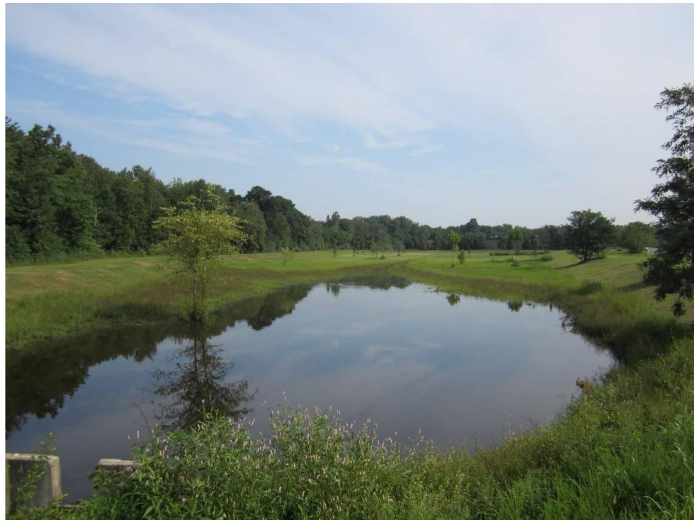
Ponding in front of outlet
