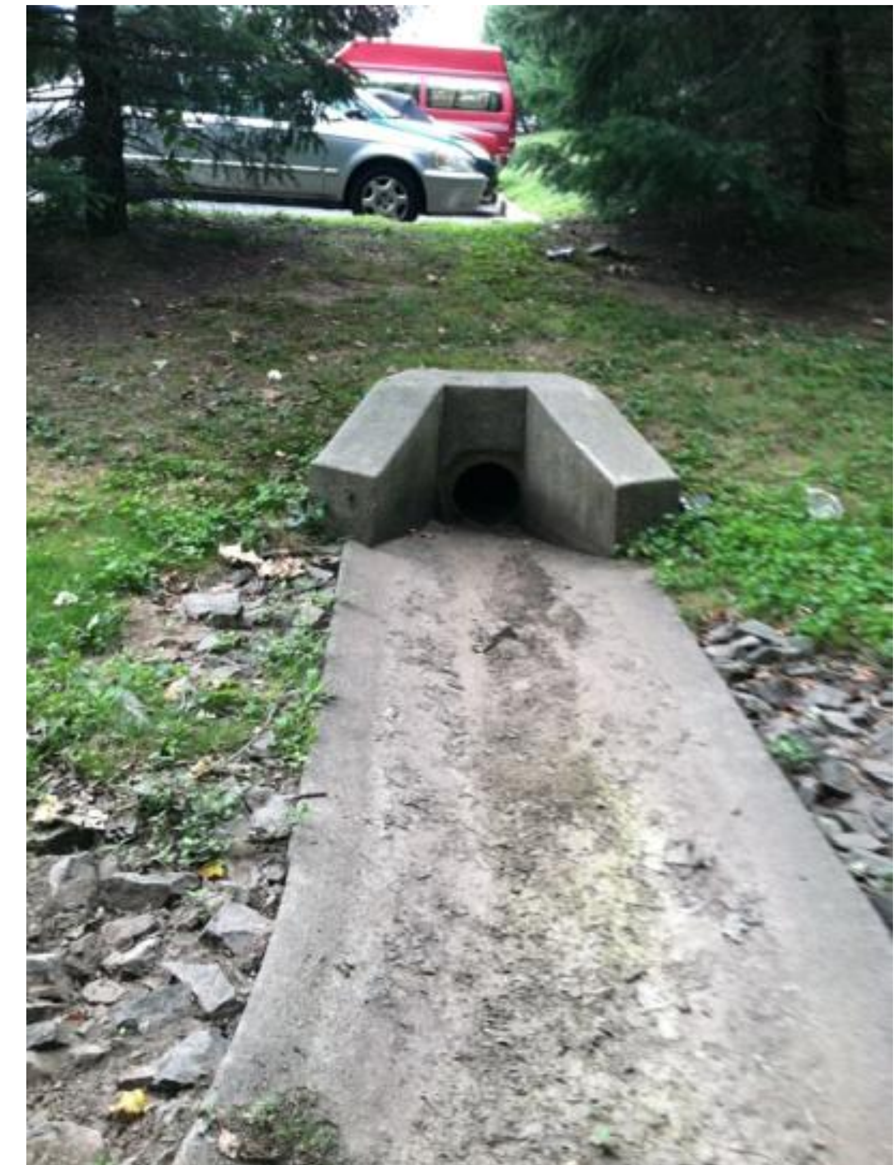
Inlet and low flow channel
