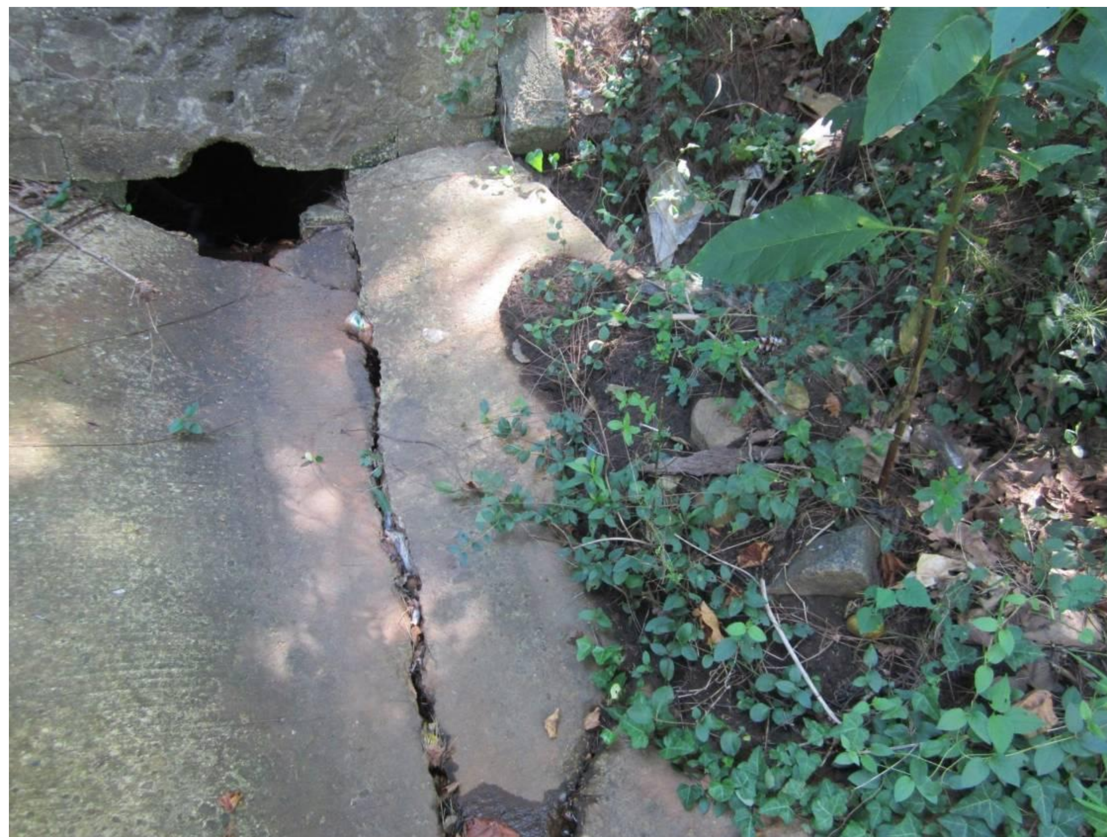
Outlet with structural damage
