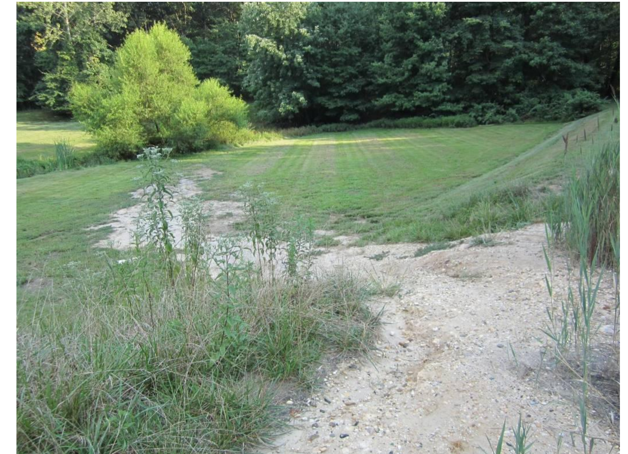
Slumping/failing basin embankment
