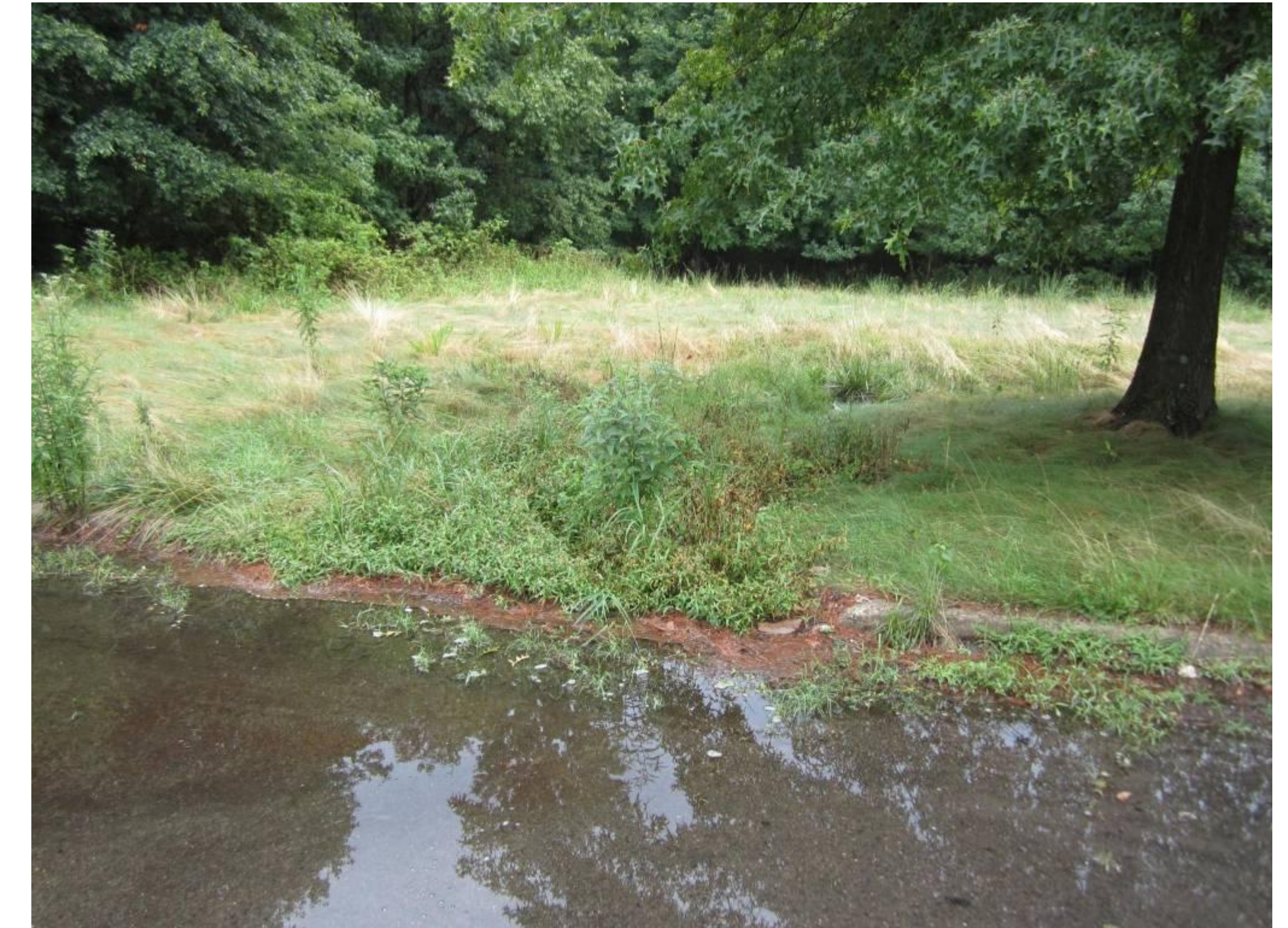
Clogged curb cut, ponding
