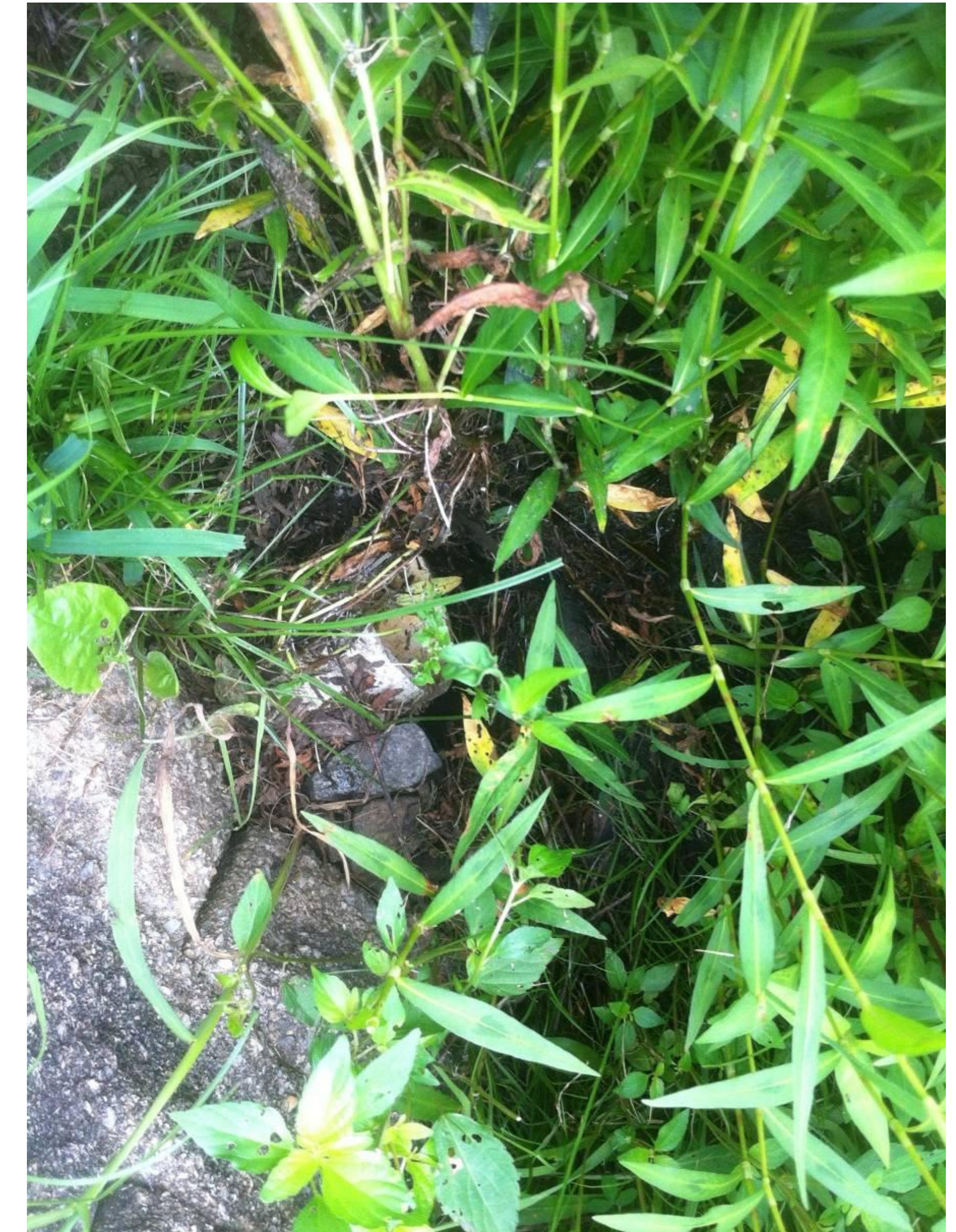
Clogged outlet orifice
