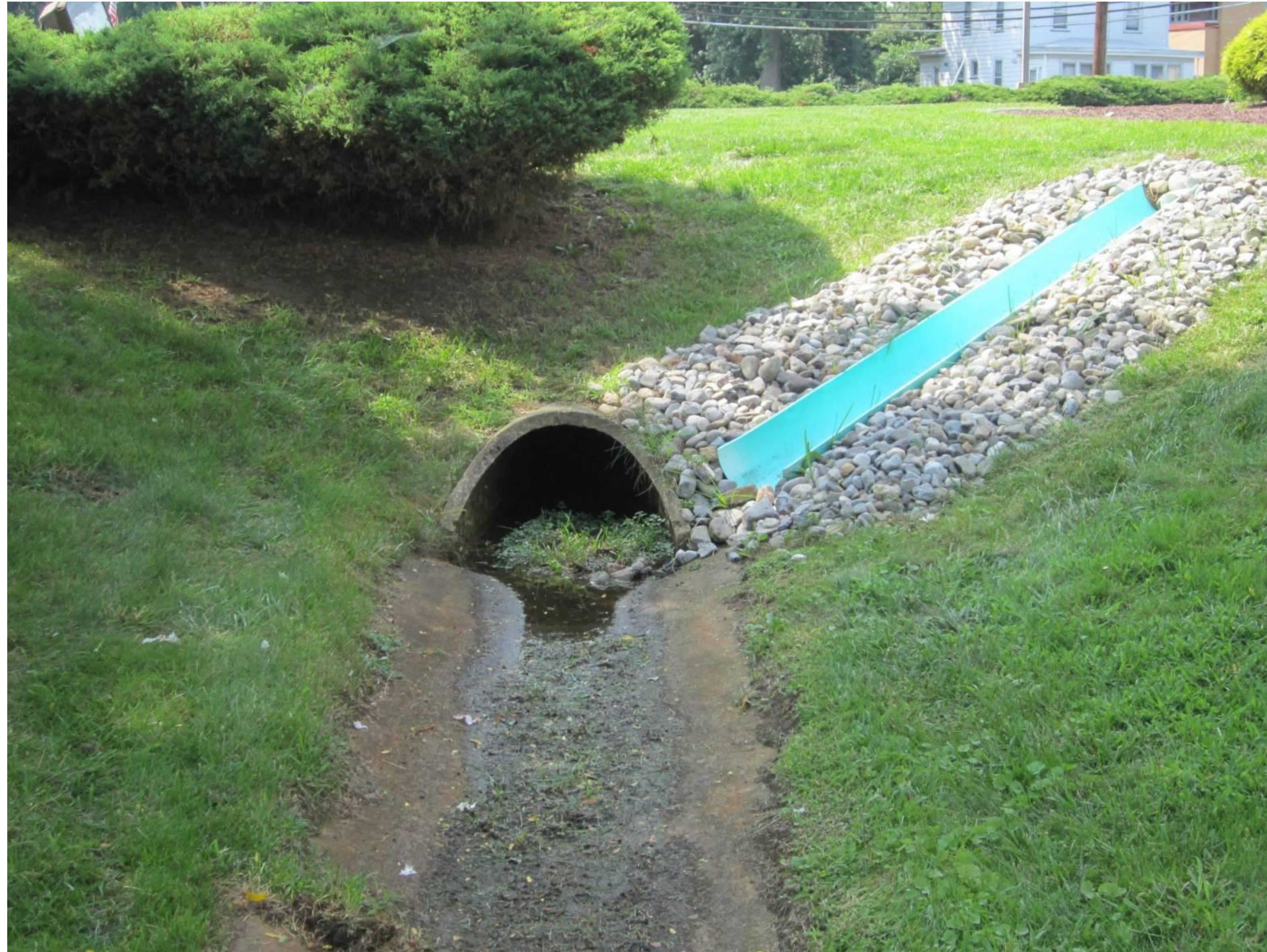
Outlet clogged with sediment
