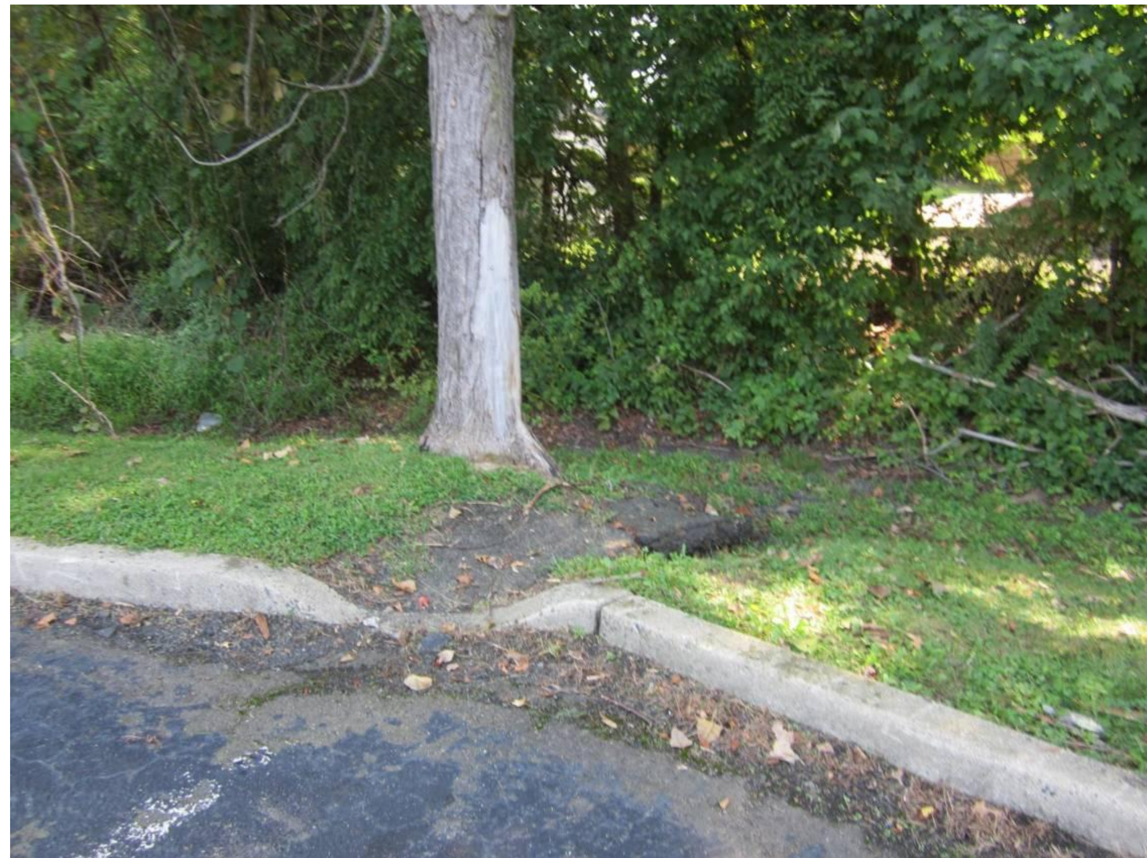
Curb cut with erosion
