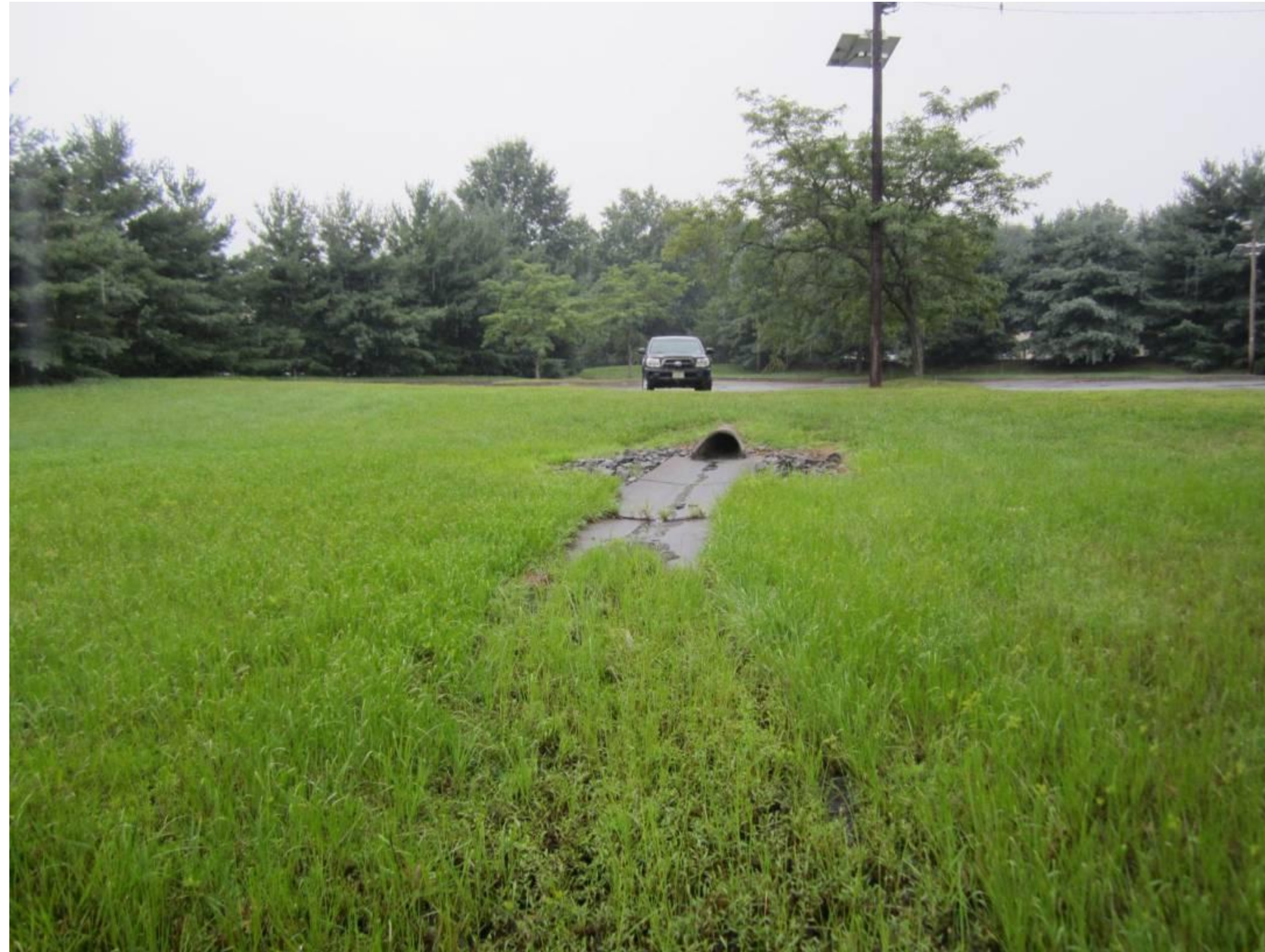
Inlet, low flow channel filled with sediment
