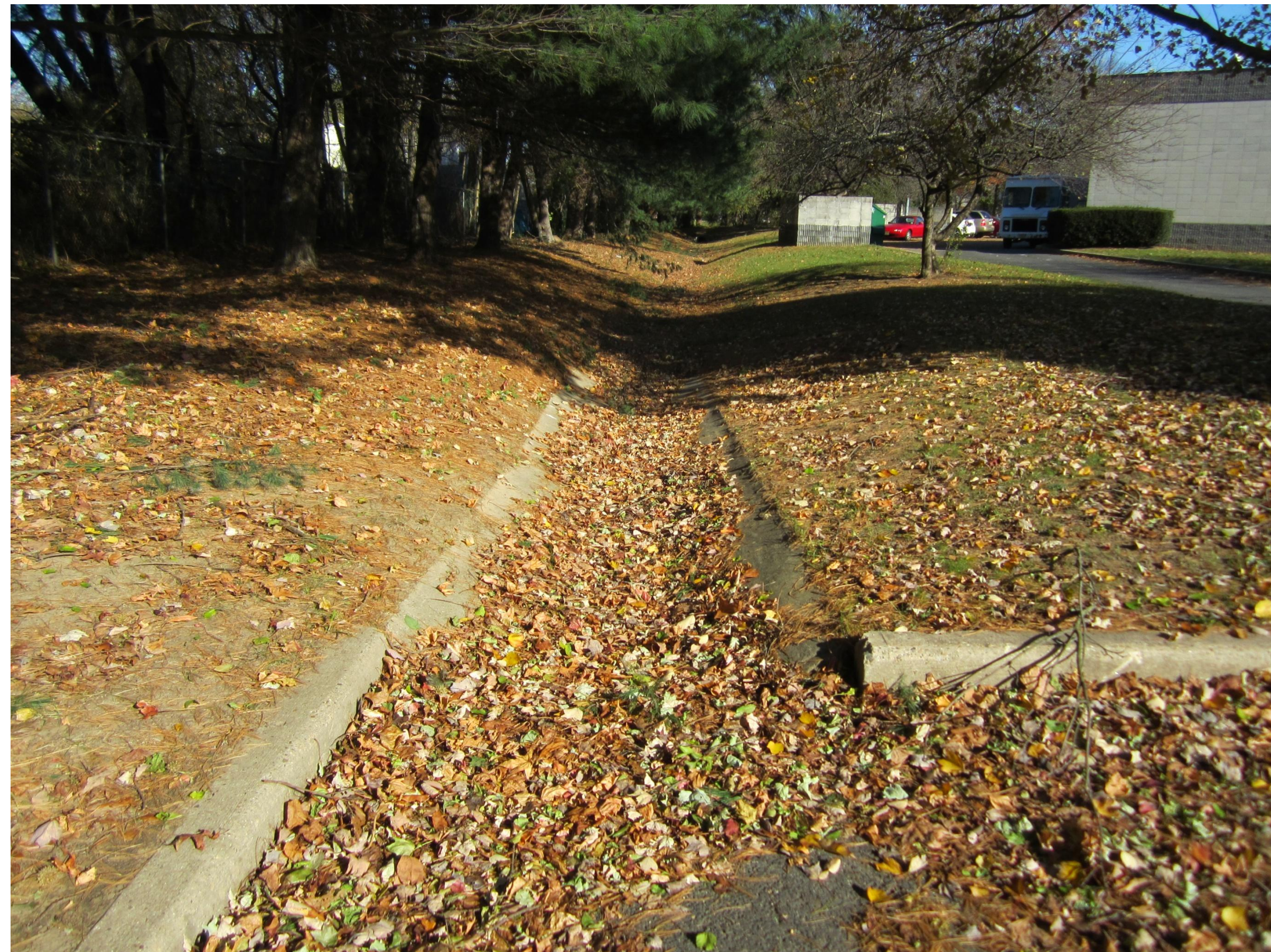
Curb cut inlet and swale
