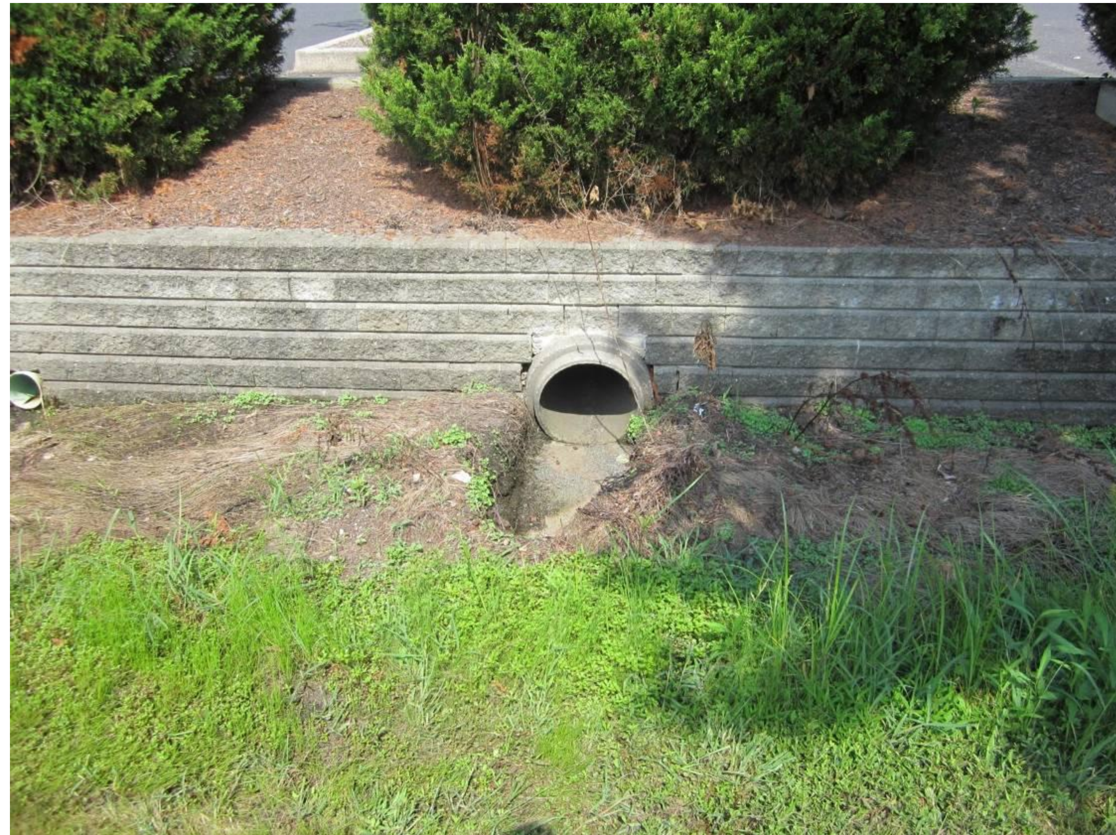
Inlet with sediment accumulation
