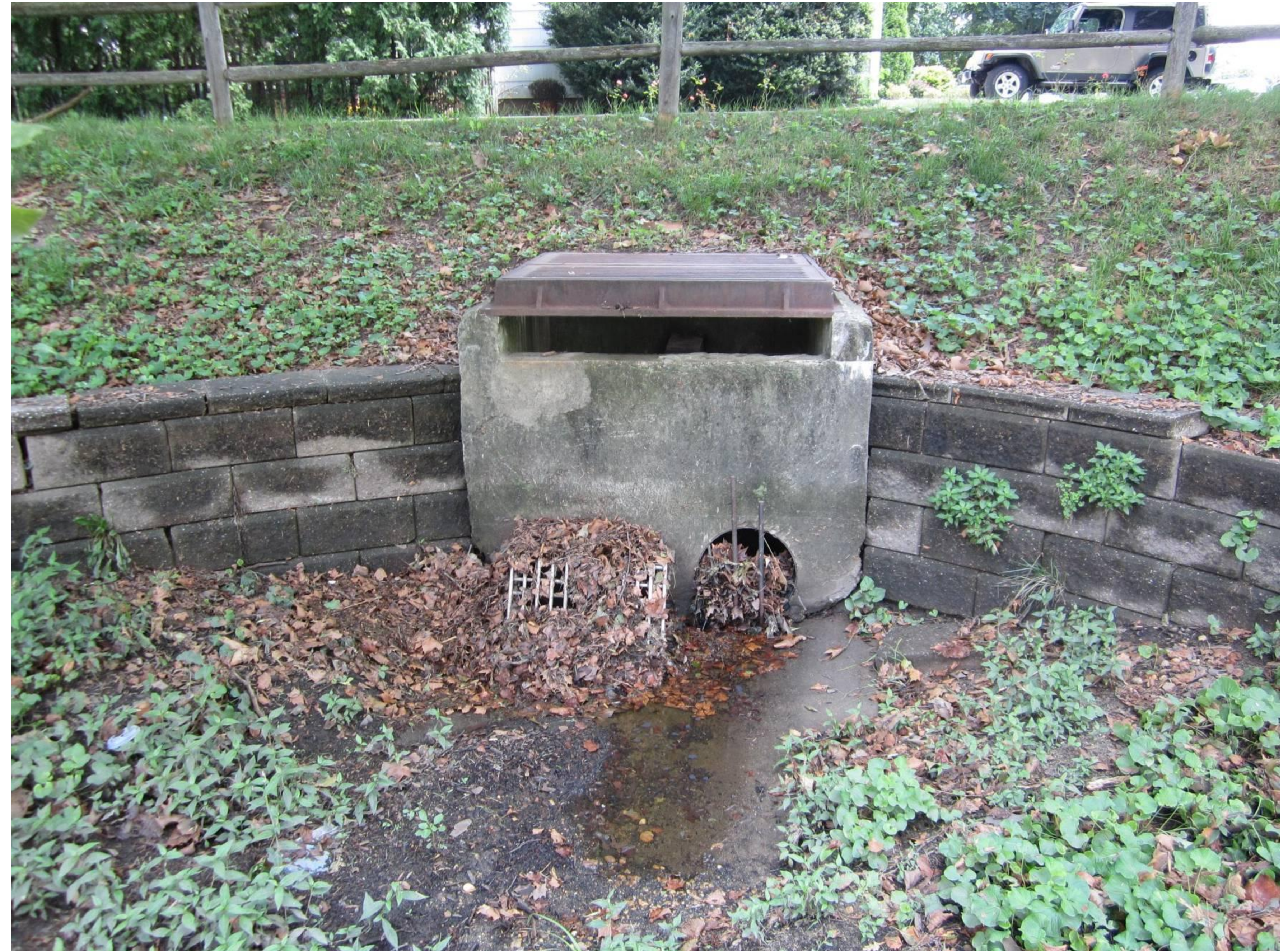
Clogged outlet structure
