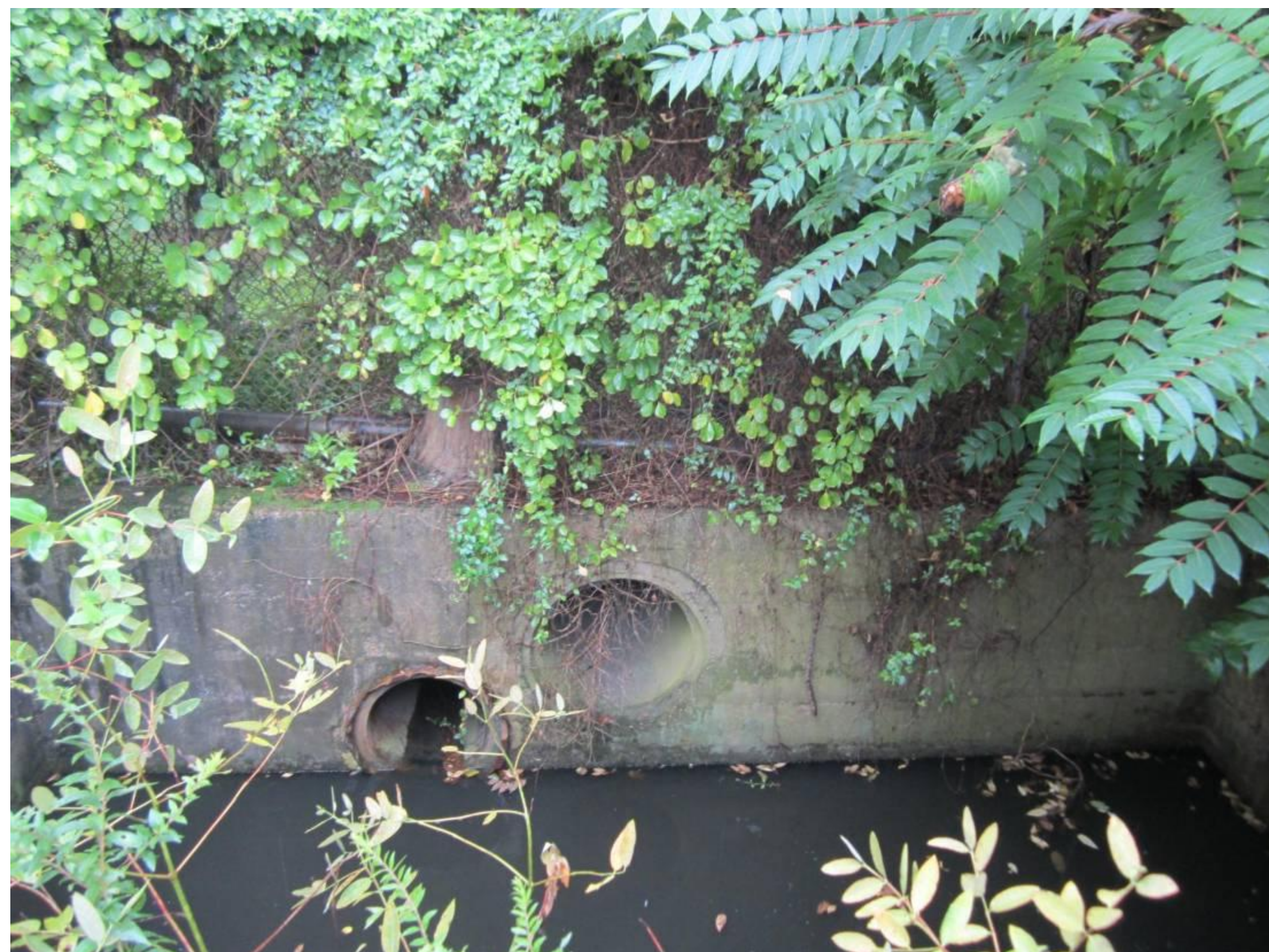
Collection for rooftop runoff
