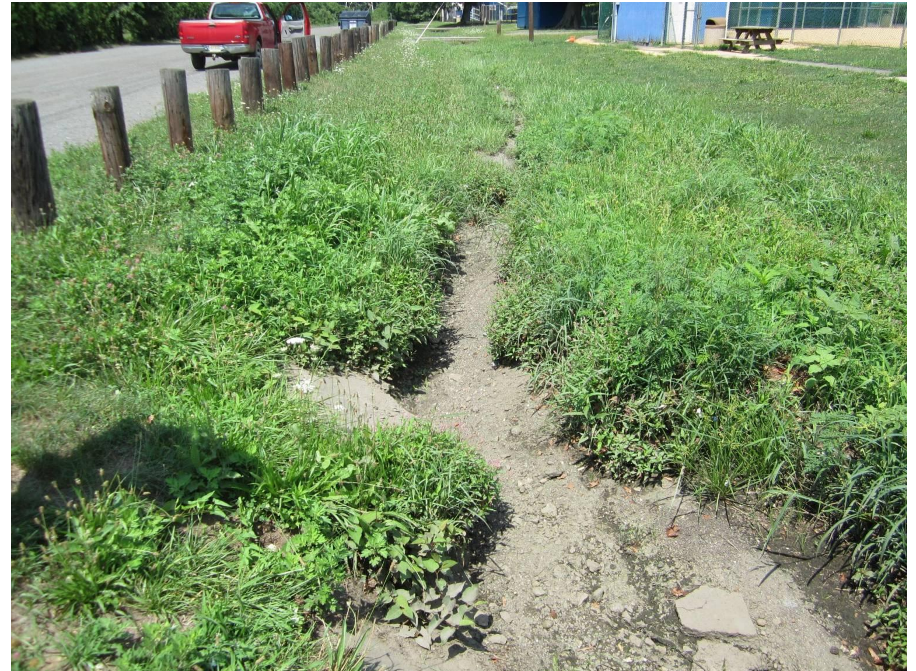
Basin bottom with erosion
