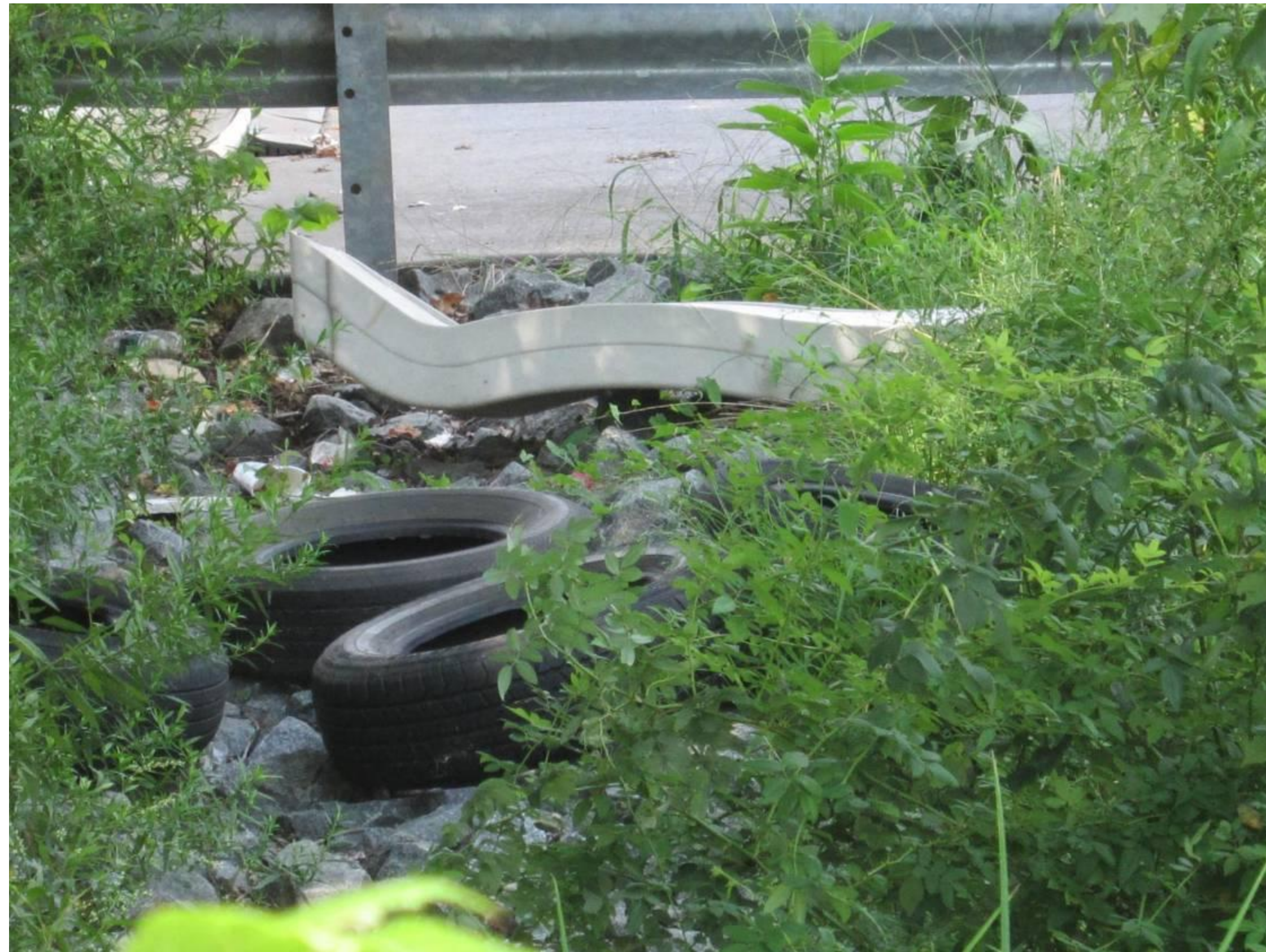
Rip rap and trash at dead end leading to basin
