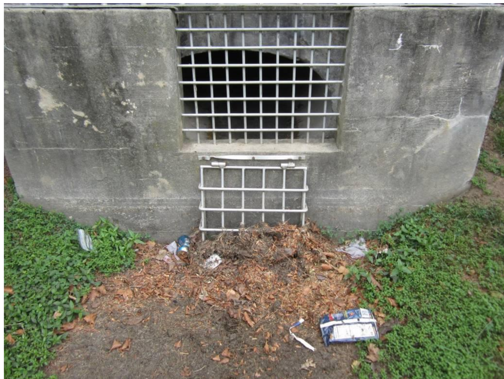
Clogged outlet grate
