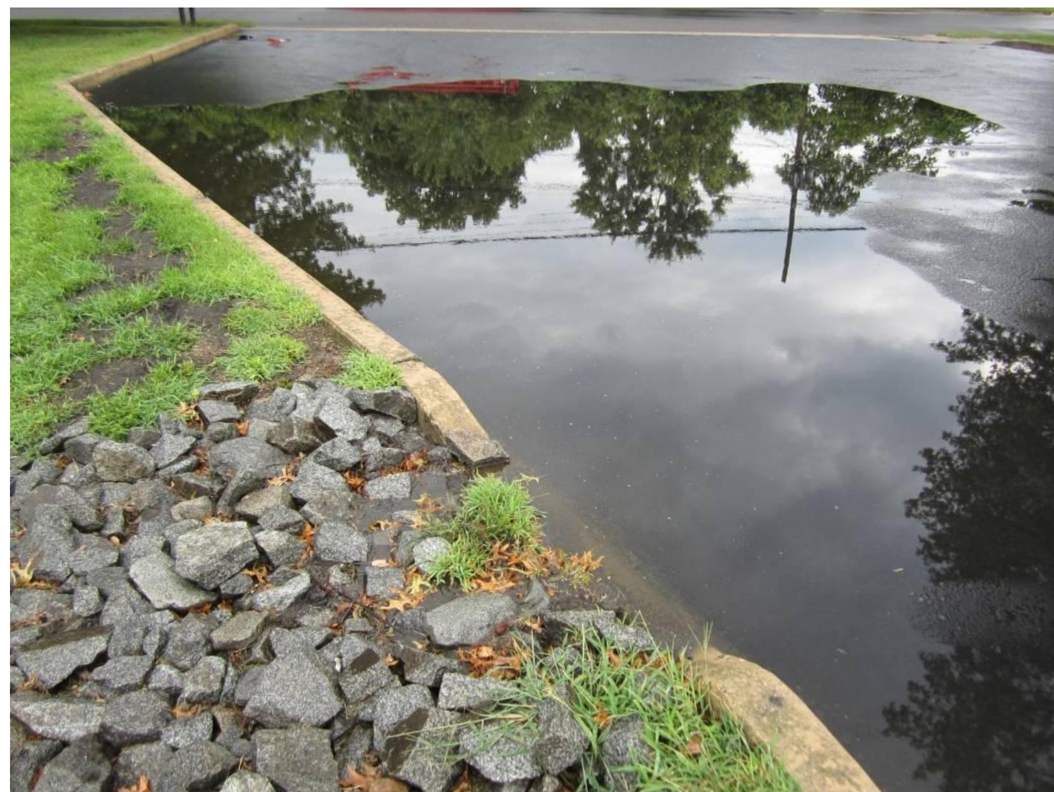
Ponding in front of curb cut
