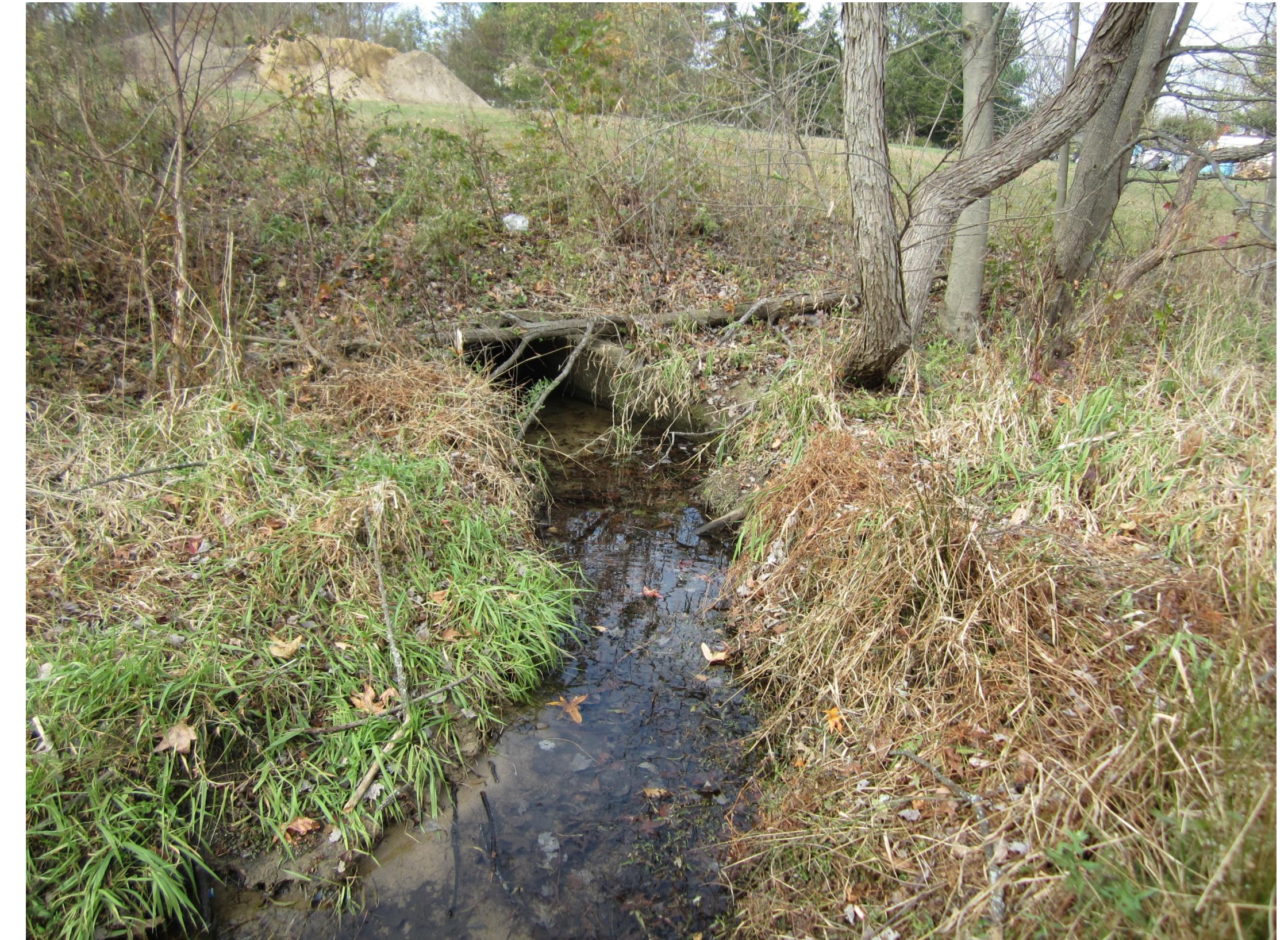
Inlet and erosion
