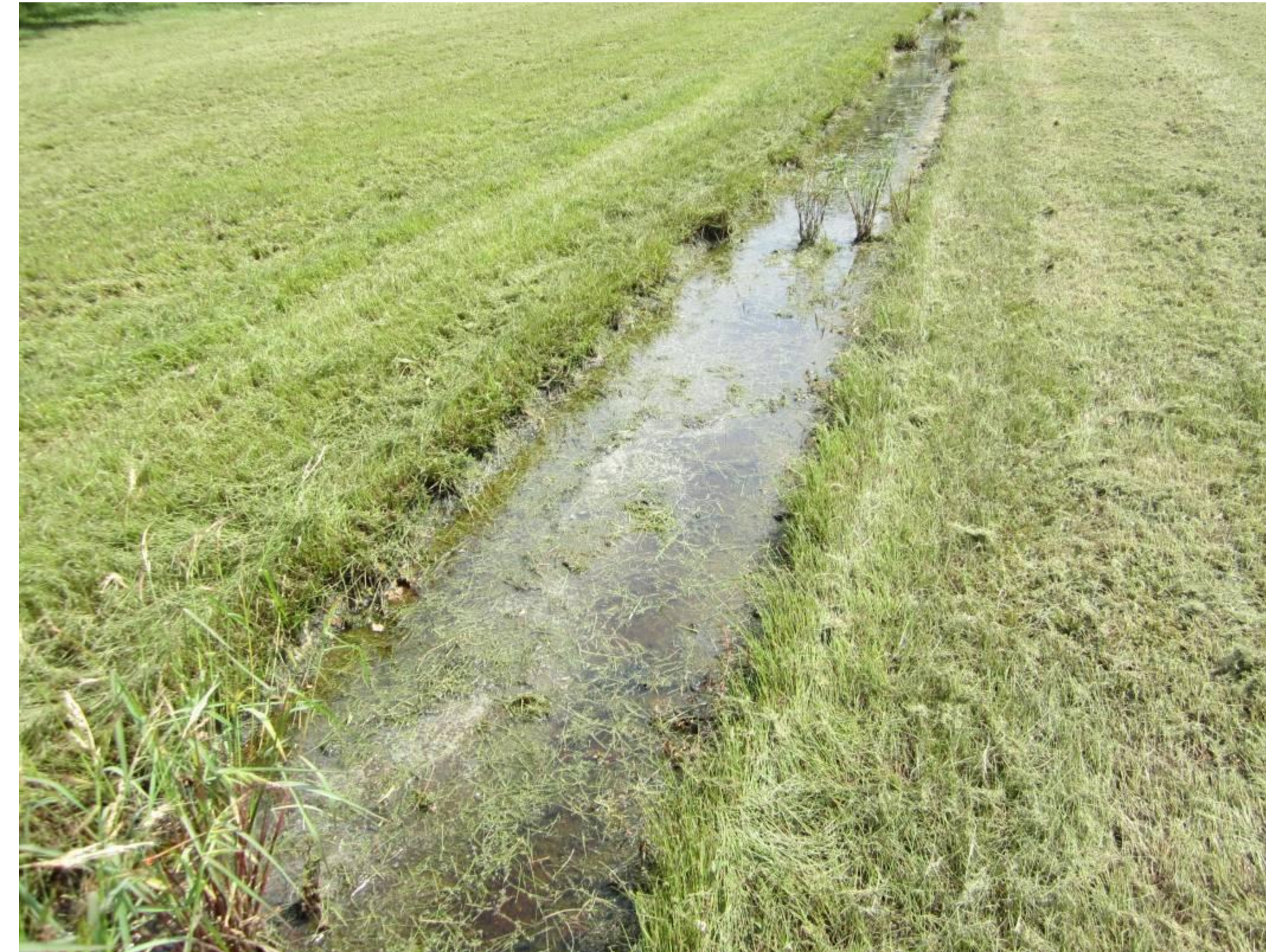
Standing water in low flow channel
