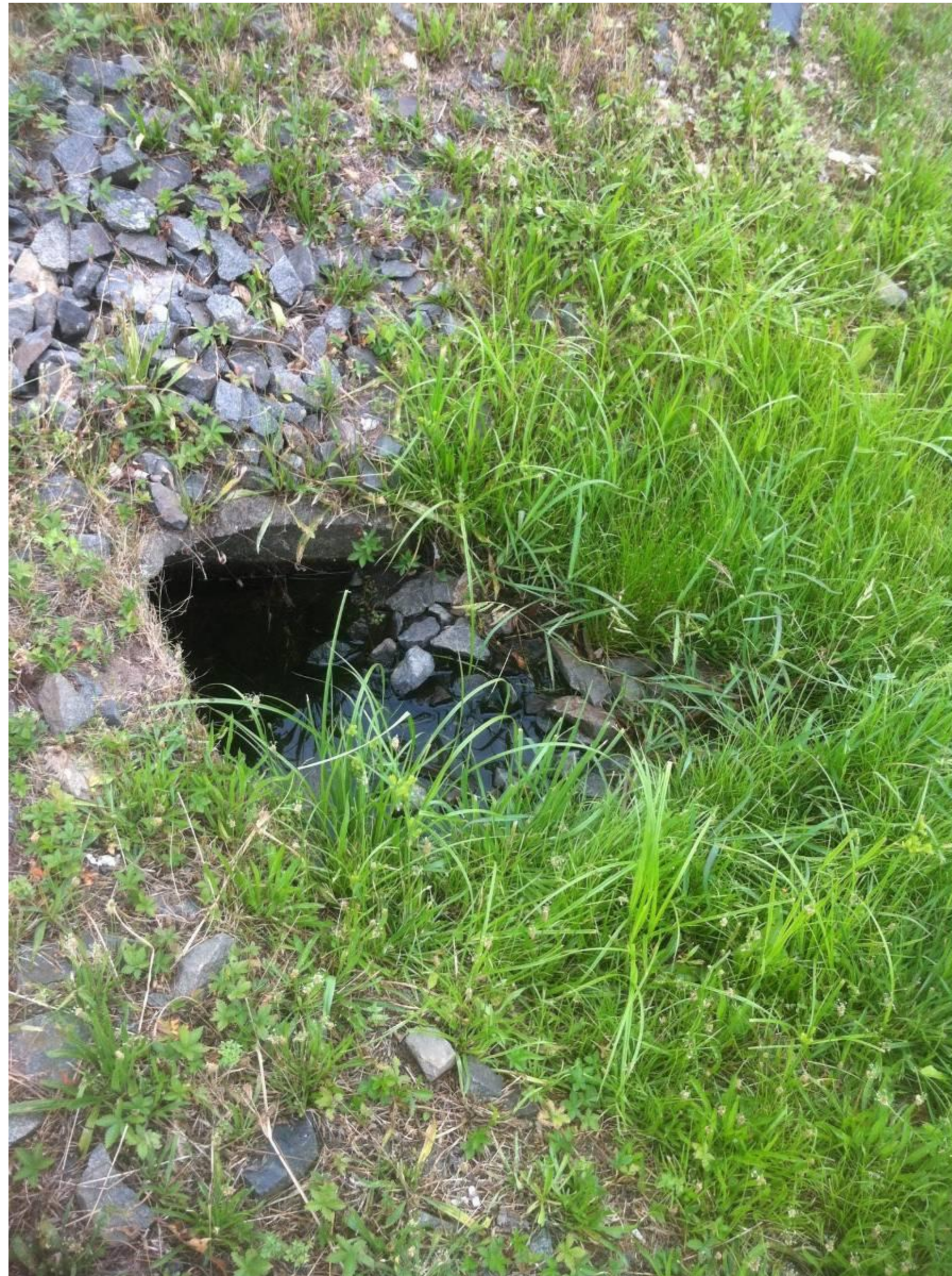
Inlet and erosion
