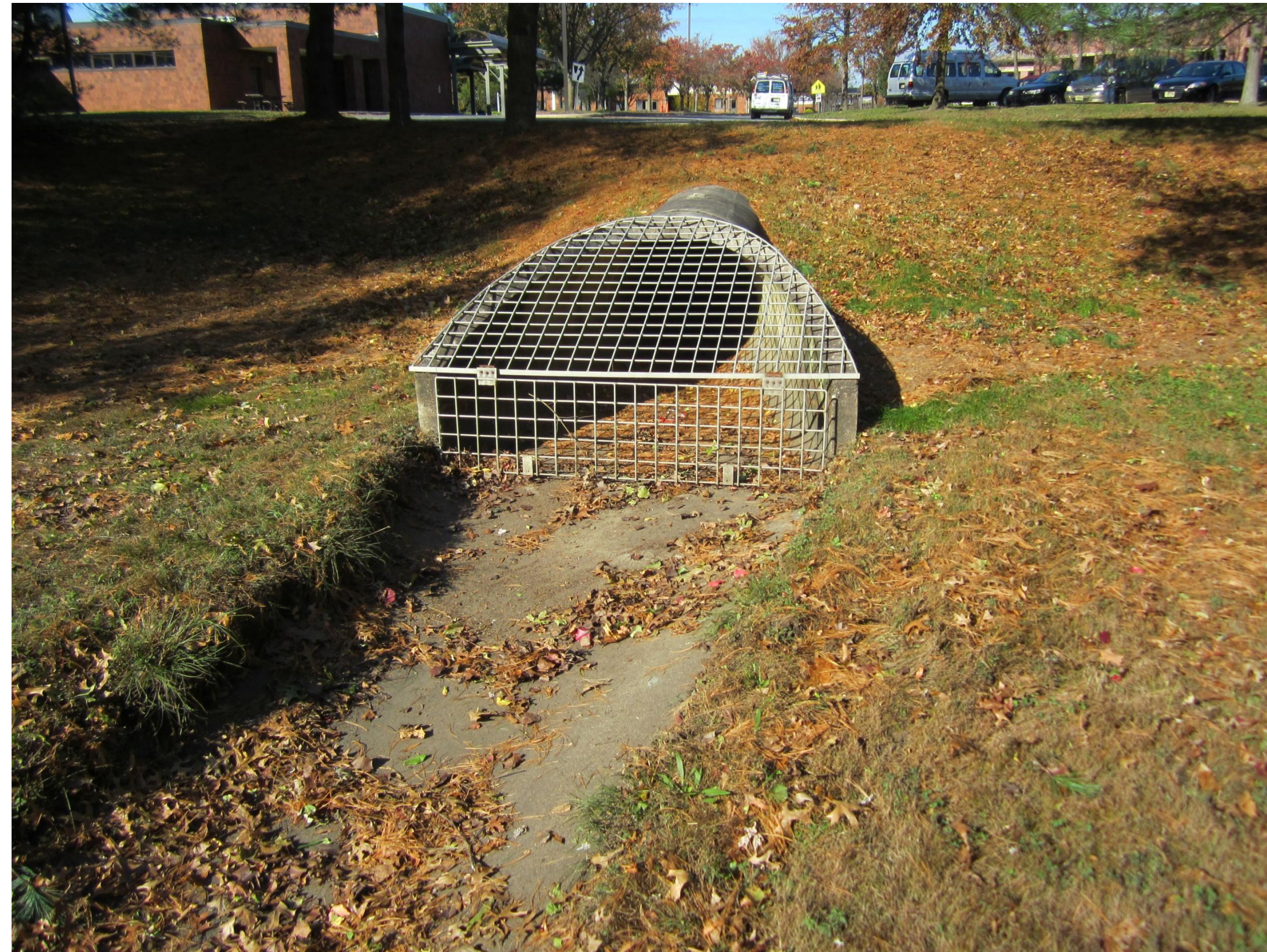
Inlet with trash rack
