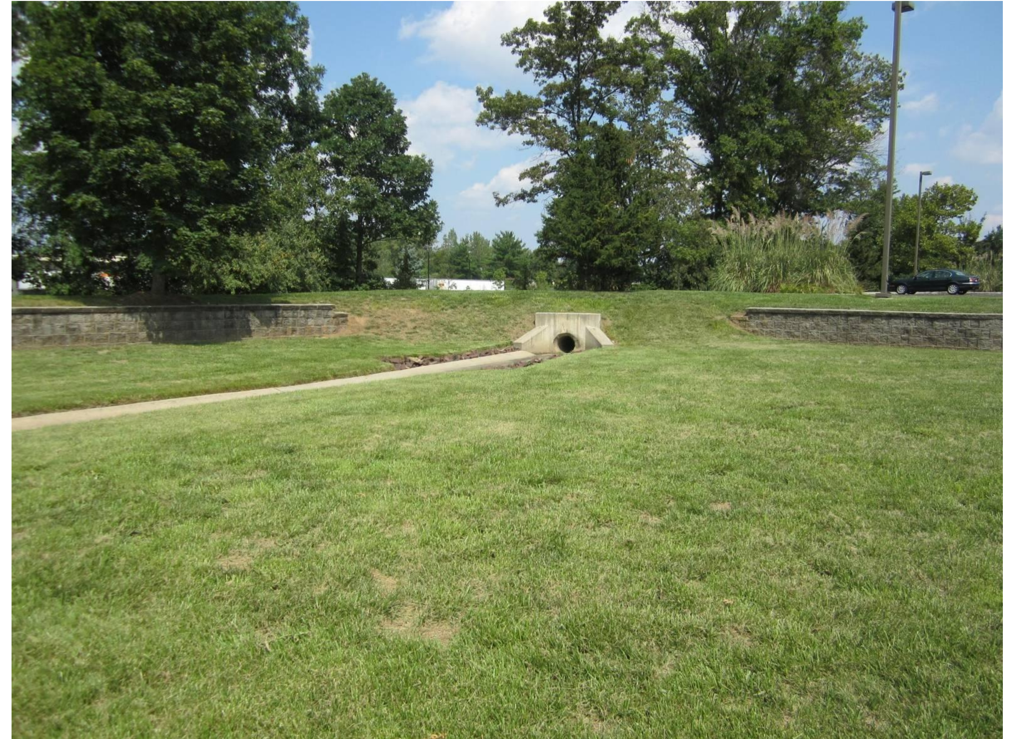
Inlet and low flow channel
