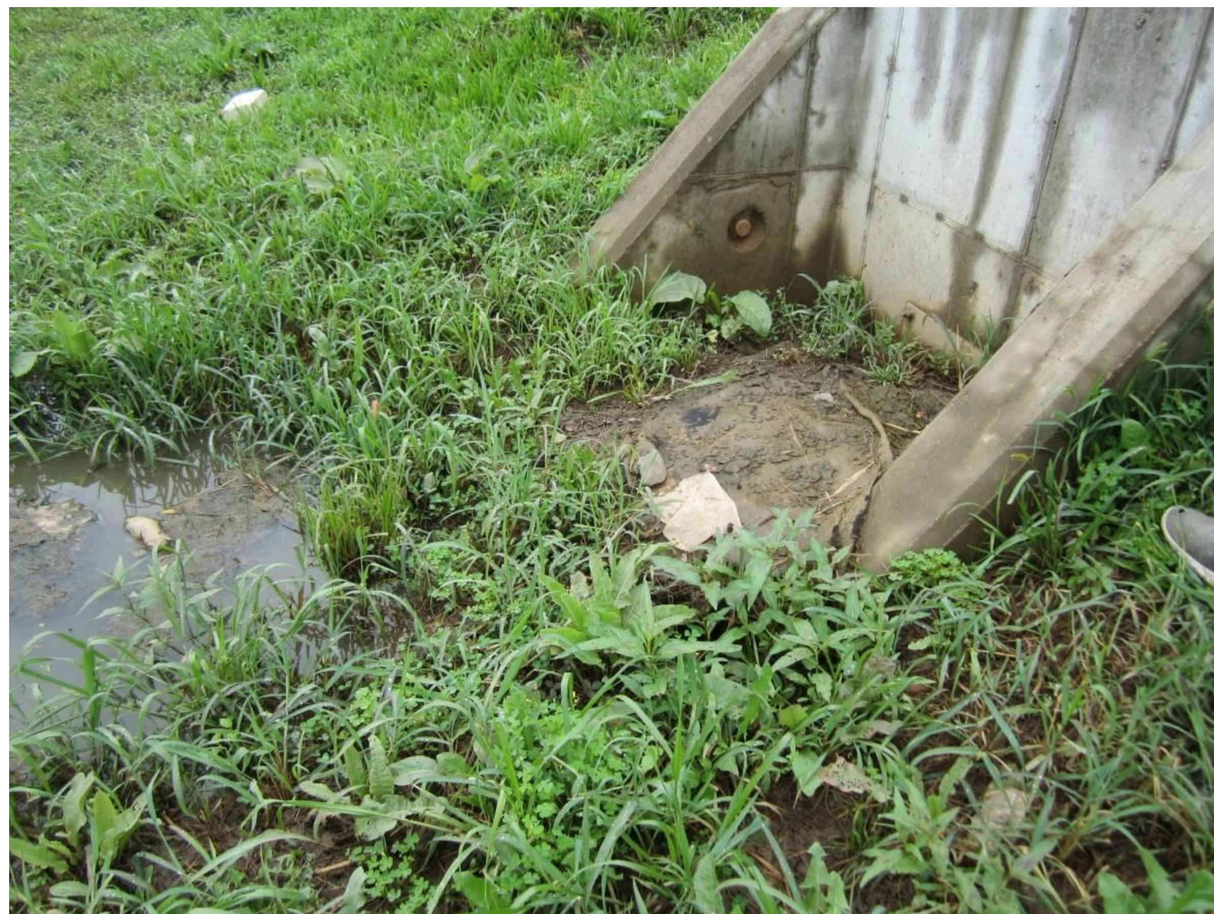
Clogged outlet orifice
