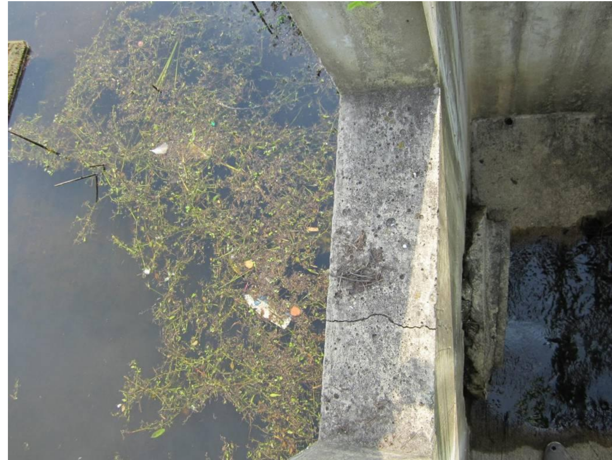
Clogged outlet structure
