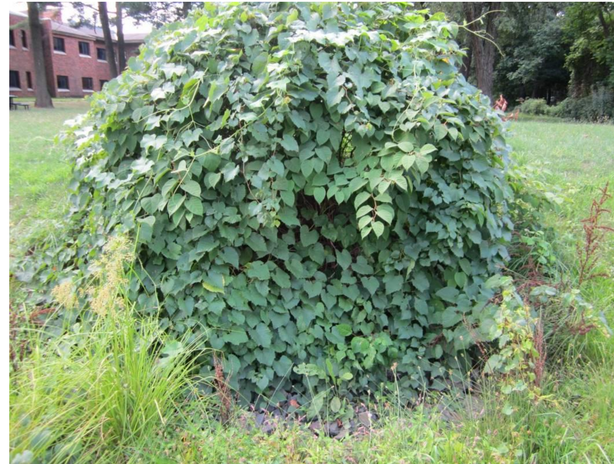
Overgrown outlet structure
