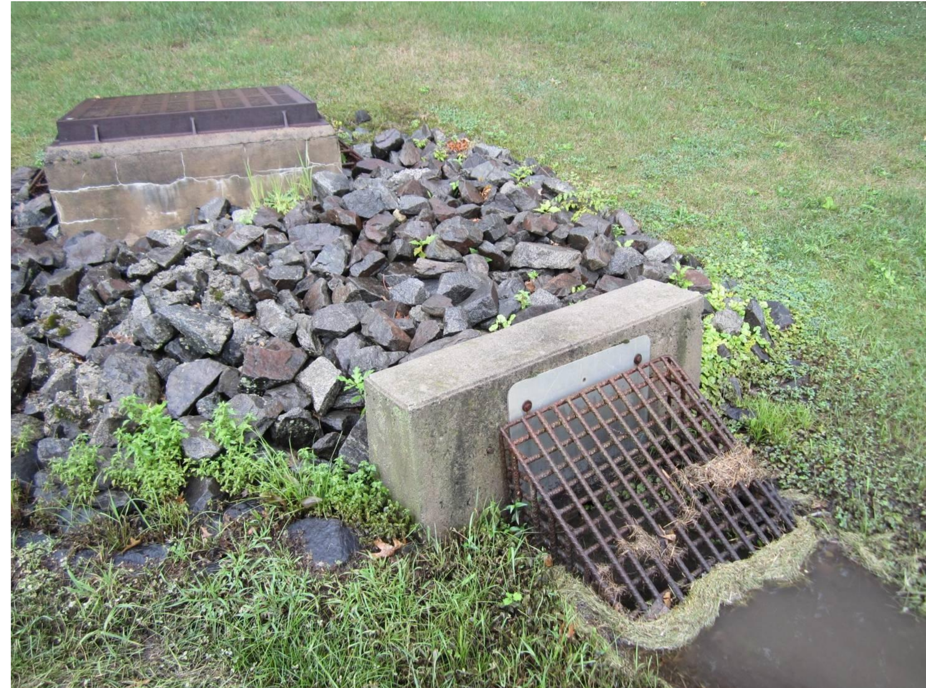
Outlet trash rack clogged with grass clippings
