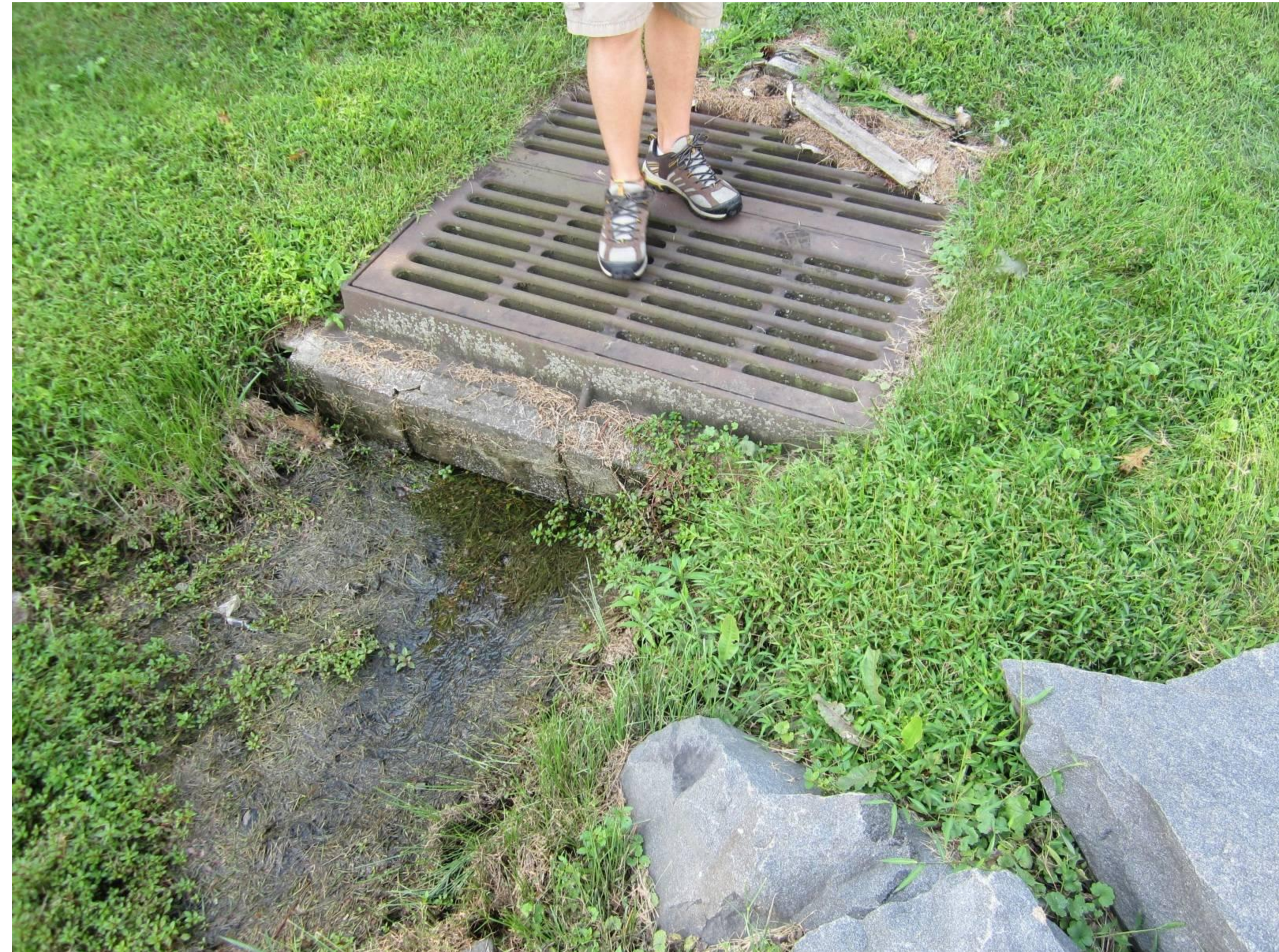
Outlet with clogged orifice
